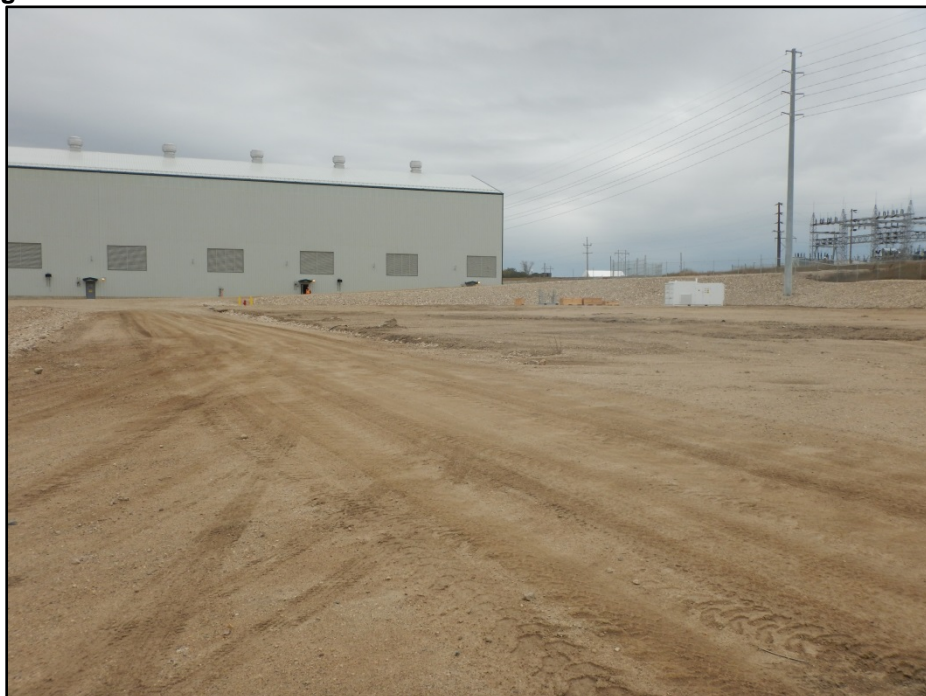
Figure 2. Former temporary workspace east of the TGP Expansion. Weed control around the site is being maintained.
