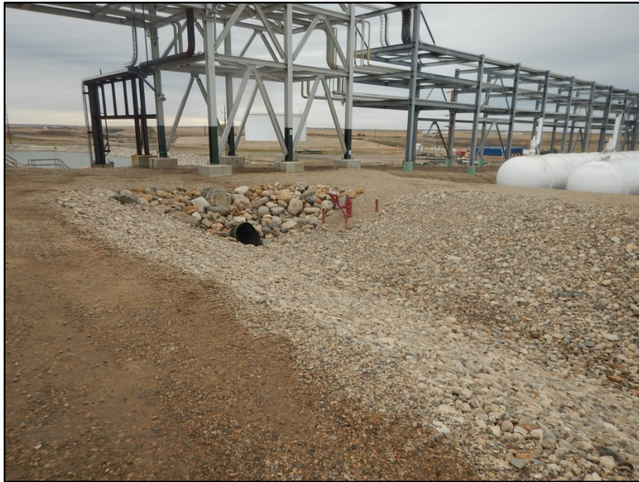
Figure 3. All drainages established within the project site have been stabilized by gravel and rock.
