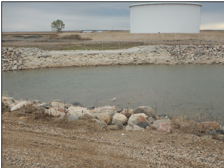
Figure 4. Sediment and standing water was observed in the stormwater pond during final inspection. The SWPPP bi-weekly reports and Hess personnel assure pond water was tested twice this year and has never overtopped.
