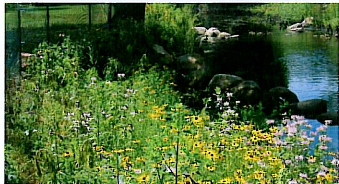
The project included narrowing and meandering the Creek, installing rock vanes and structures, stabilizing the streambanks with live stakes, and planting a native buffer.
