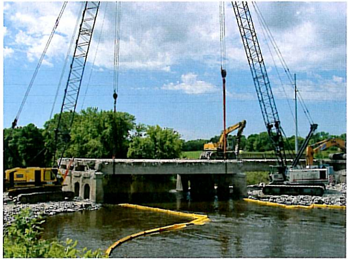
Construction of the Trunk Highway 12 Crow River Bridge in Delano, MN. As Delano's City Engineer, Wenck participated on the inspection team and provided a wide-variety of additional support in everything from tank excavation to community relations.
