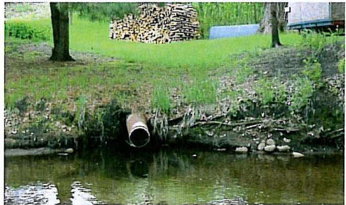
Prior to restoration the Creek was overwide, with a flat bottom and eroding banks. Turf grass was maintained up to the edge of the Creek.
