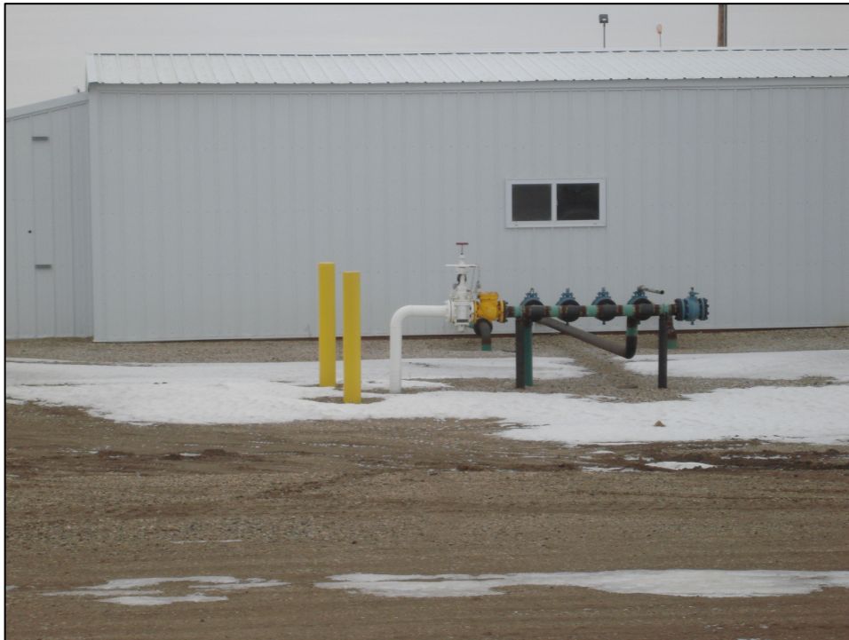
Photo 14. Direction: East. The white pipe and valve was installed as part of the PU-10-130 project, the additional pipes, valves, and building are installed by other companies to connect to the Enbridge system.
