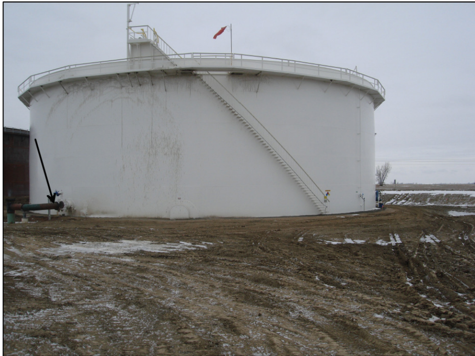
Photo 12. Direction: Northwest. Arrow showing the 10 inch line that serves as the inlet and outlet of the rehabilitated tank.
