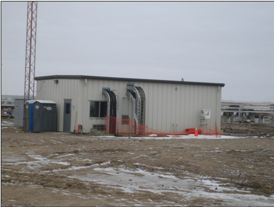
Photo 7. Direction: Southwest. This building contains the controls and variable frequency drives, the wire trays and wires are shown entering the building. The tower on the left side of the building for SCADA telemetry.
