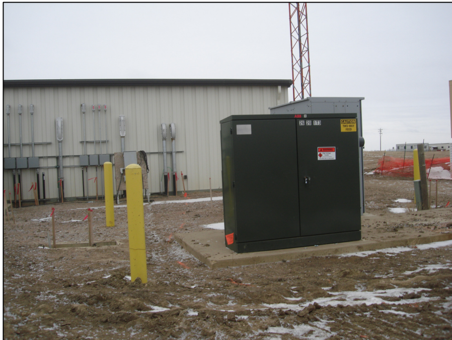
Photo 6. Direction: Northeast. Photo showing the new electrical transformer that was installed on this project. The building in the immediate background contains the controls and variable frequency drives.
