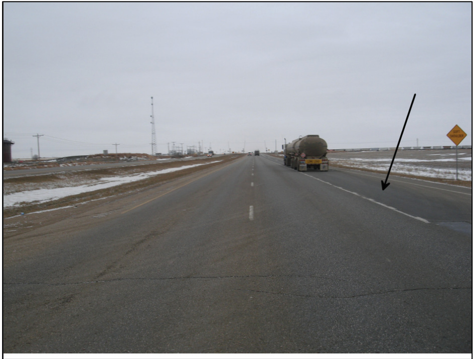
Photo 2. Direction: West. Arrow showing the acceleration lane for westbound traffic leaving the site at the intersection of 296 th St. and Highway 2. Photo also shows road ditches have been graded and reseeded.
