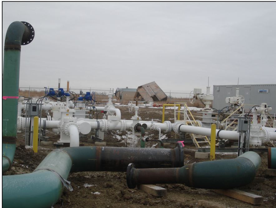
Photo 10. Direction: South. The piping and valves painted white are part of the PU-10-130 project, all other piping and disturbances are part of a different project that is currently under construction.
