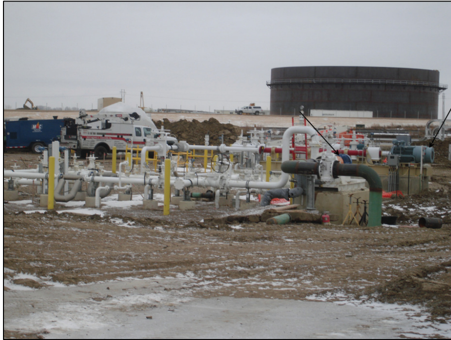
Photo 9. Direction: Southwest. Arrow on the left is pointing to the 50 Hp booster pump and arrow on the right is pointing towards the centrifugal pump that replaced the two positive displacement pumps.
