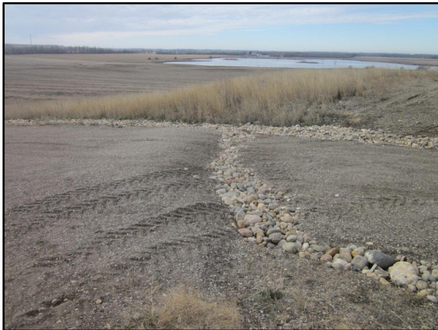
Photo 14. Direction: Southwest. Access road near Turbine 282 where an erosional cut had been filled in with rocks to prevent further erosion, while allowing continued natural drainage flow.
