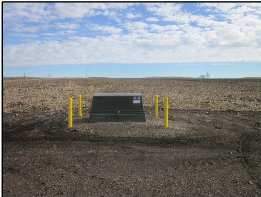
Photo 8. Direction: East. Junction box JB102 along 21 st St SE showing typical conditions. Cement bollards and gravel were in place around the box with no indication of erosion or weeds. Safety warning signs were in place.
