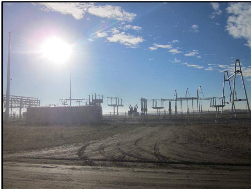
Photo 2. Direction: South/Southeast. New substation built for Ashtabula III.
