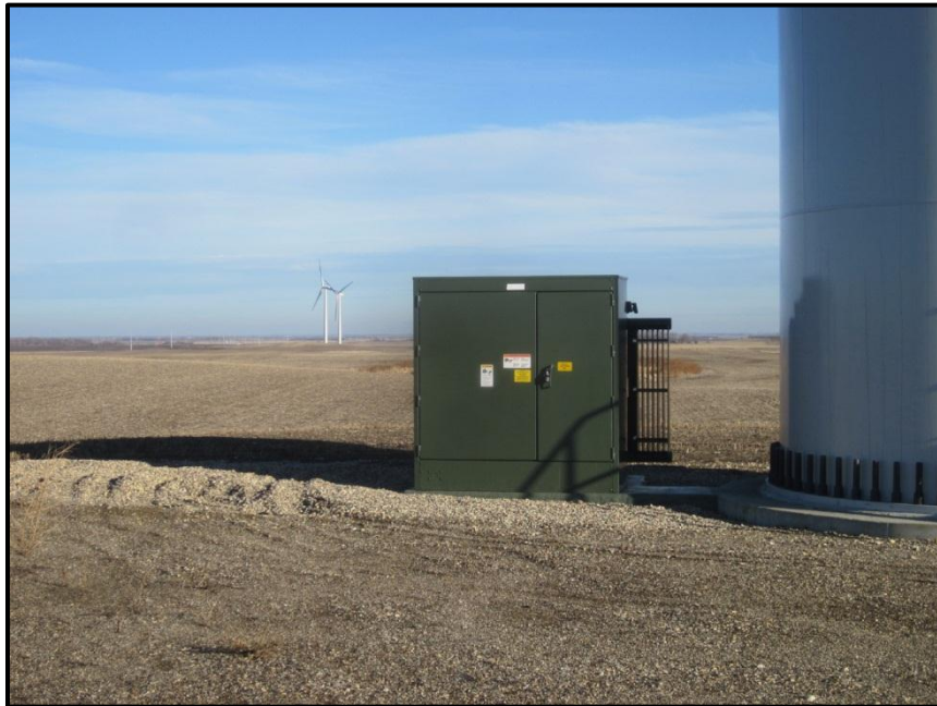
Photo 22. Direction: East. Base of Turbine 264, showing extra gravel containment underneath the pad-mounted transformer to help prevent spills or impacts to the adjacent waterway.
