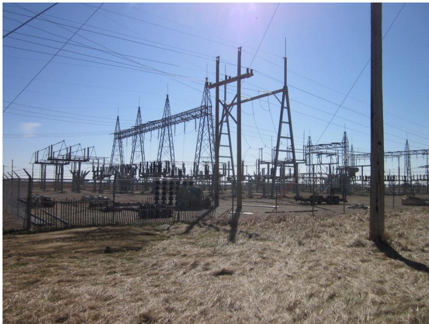
Photo 4. Direction: Southeast. Ellendale substation.
