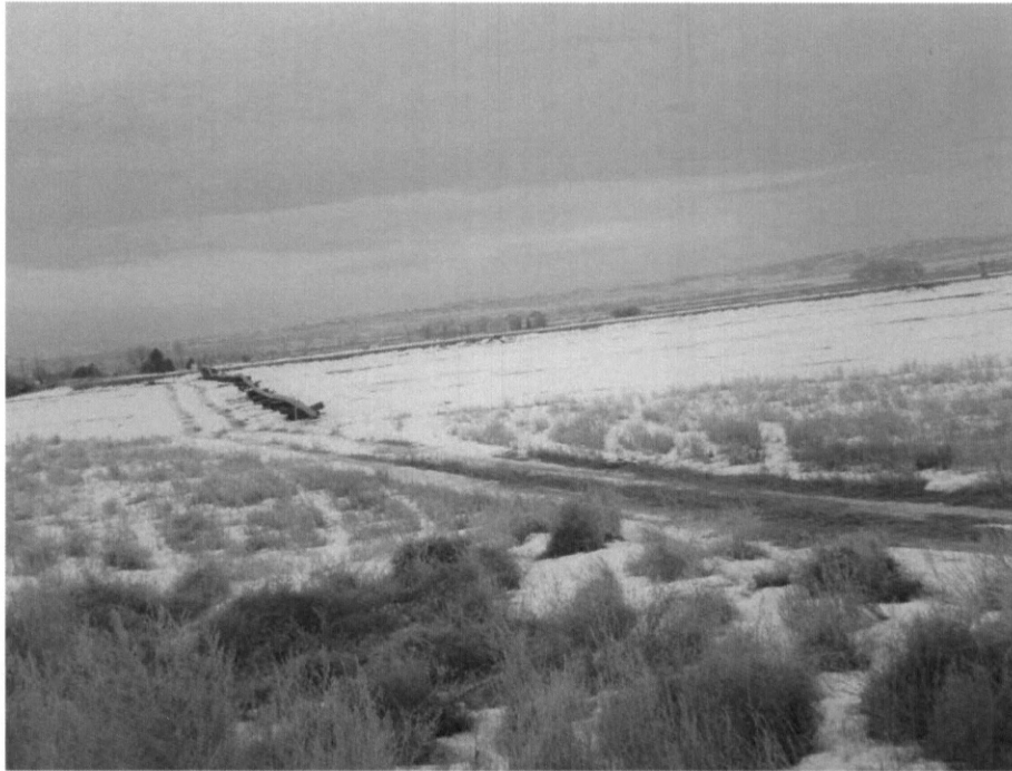
Photo 6: Looking east from 158 th Ave, ROW staking present, pipe stringing almost complete in prep for HDD of Yellowstone River.
