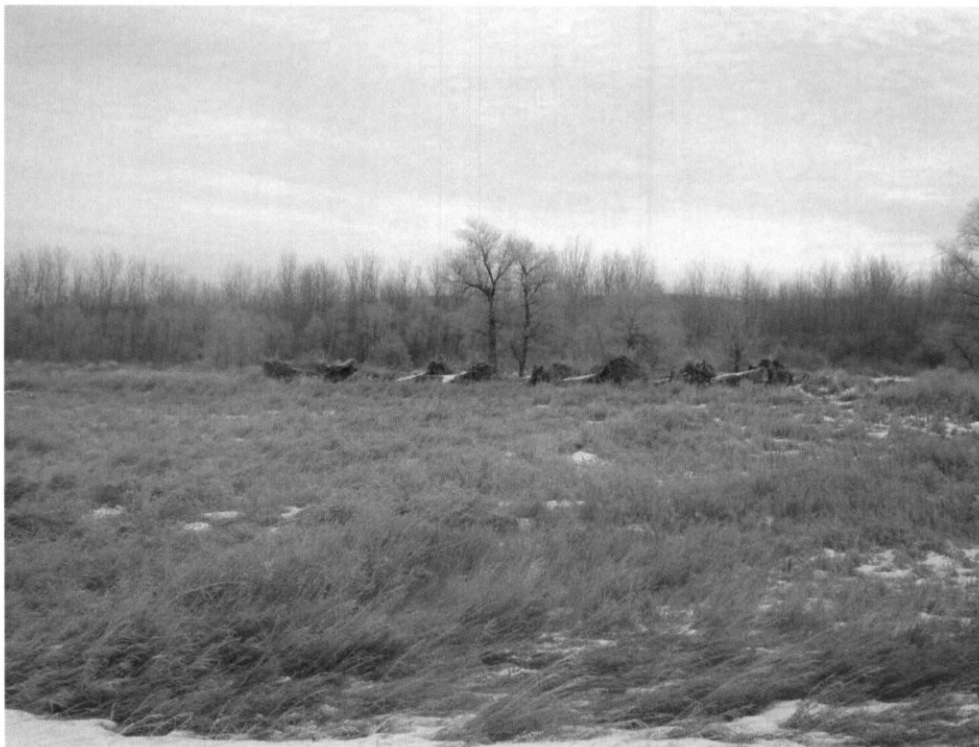
Photo 5: Looking west from 158 th Ave towards Yellowstone River, ROW staking not present, prep for HDD of river being conducted on East side of road, see Photo 6.
