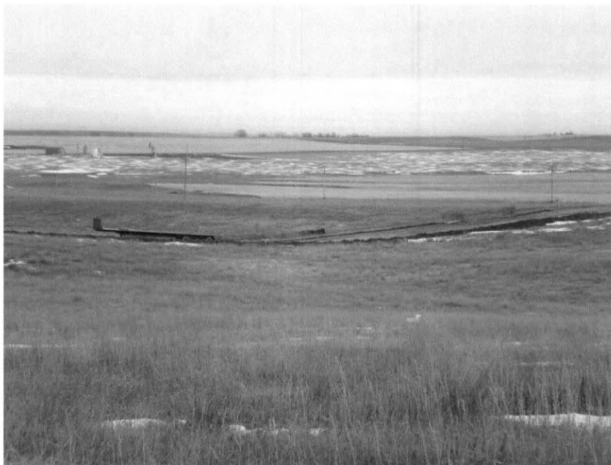
Photo 2: Looking north at ROW from County Rd 16 at 1 st drainage way crossing, not presence of silt fence on the north side of the ROW and the orange safety fence to mark the location of other pipelines crossing the construction ROW. The pipe has been placed in the ground at this location.
