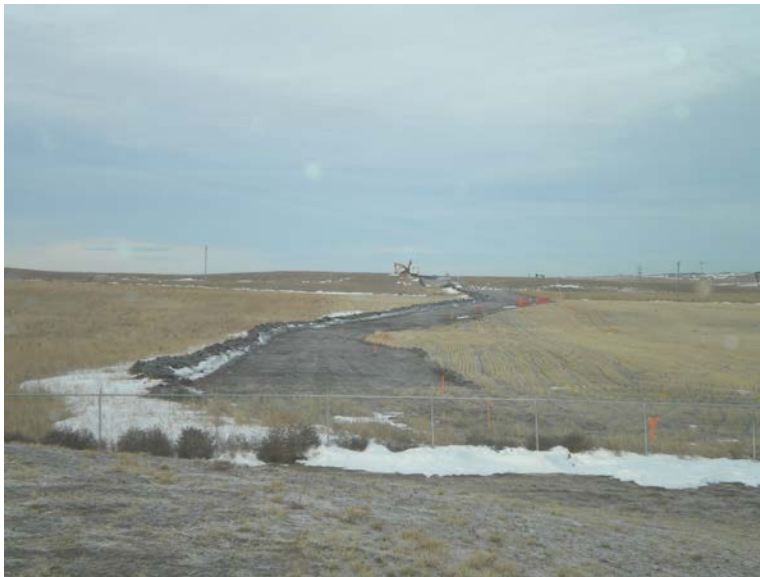
Photo 1: Looking west from Hiland Operating Plant at Project ROW, at this location pipe has been placed in the ground however topsoil has not been replaced, also ROW staking is present
