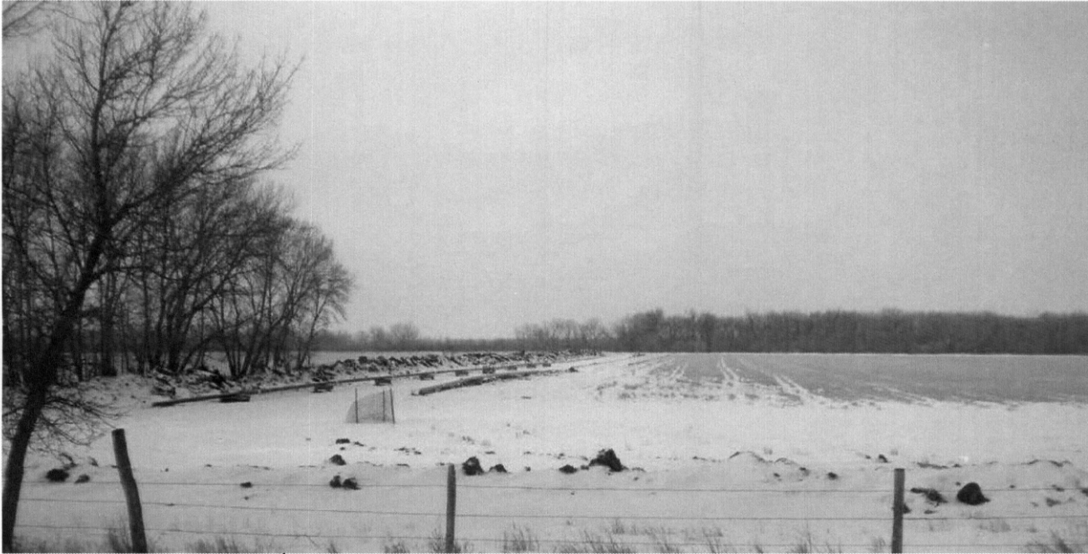
Photo 4: Looking west from 157 th Ave. NW at pipe strung for installation up to eastern side of Yellowstone River and tie-in into Yellowstone River HDD.
