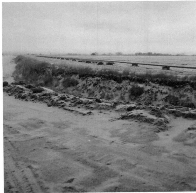
Photo 3: Looking east at pipe strung for HDD of irrigation channels and existing creek and ditches.
