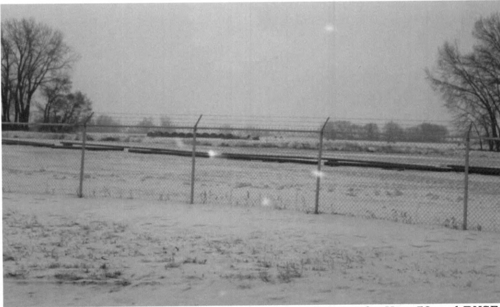
Photo 2: Looking south from Hiland Rail Terminal at pipe strung for Hwy 58 and BNSF Railroad HDD and installation of pipeline into facility.
