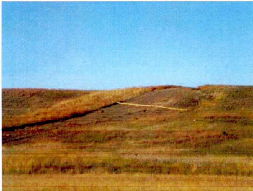
Image 5: Looking back at ROW in Section 31, erosion control measures properly placed and in good working order, regrowth of vegetation is underway. Continue to maintain erosion control measures until re-vegetation reaches 70%.
