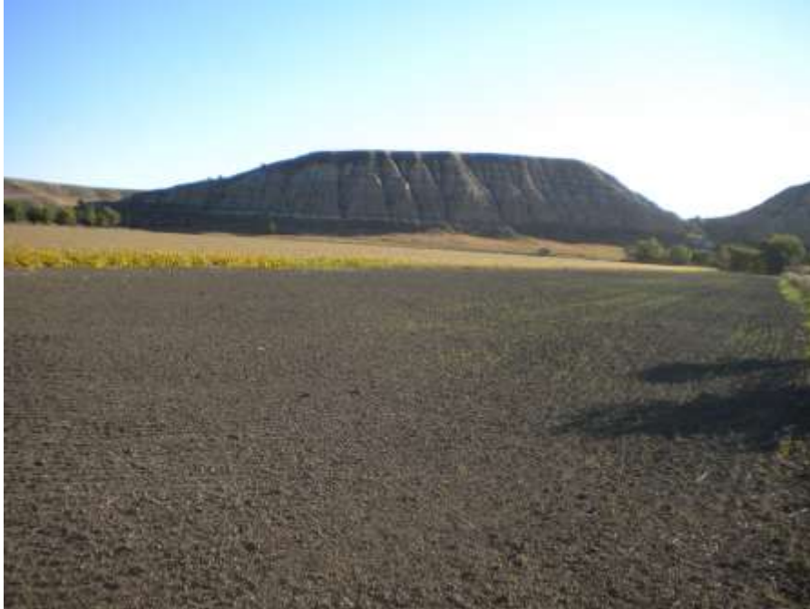
Image 4: Entry point for Yellowstone River HDD, area has been returned to agricultural use.
