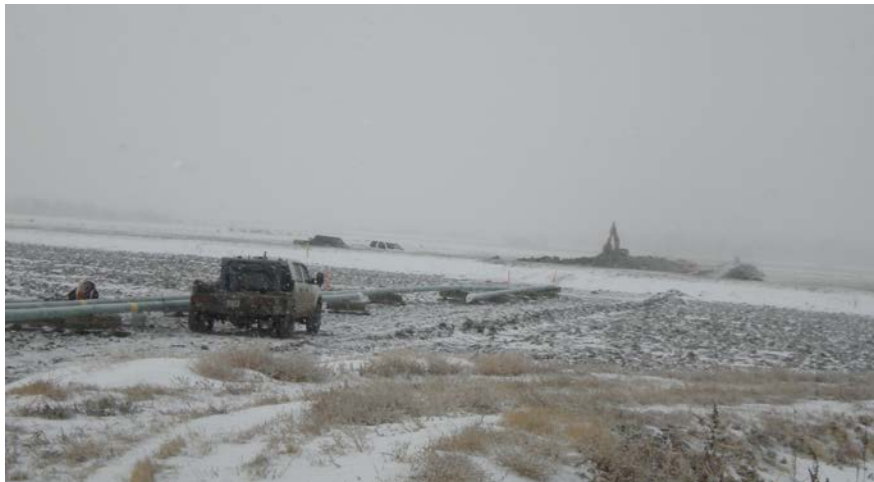
Photo 1: Looking southwest from 36 th ST NW at Project ROW, notice pipe strung in preparation installation via open trench method.
