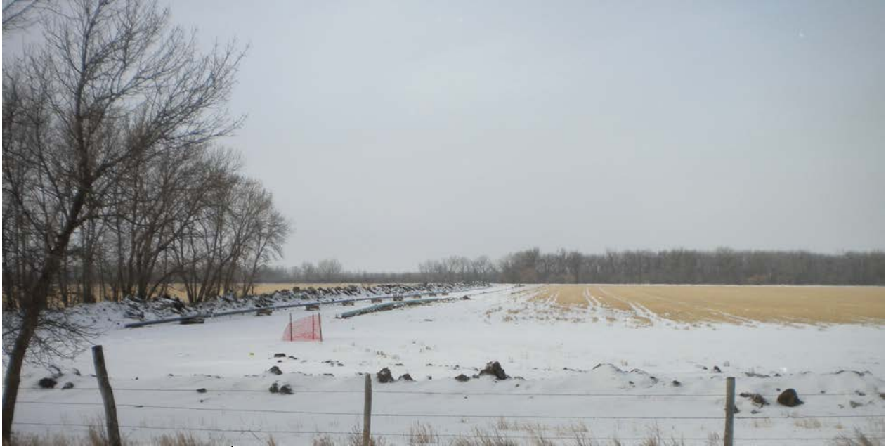
Photo 4: Looking west from 157 th Ave. NW at pipe strung for installation up to eastern side of Yellowstone River and tie-in into Yellowstone River HDD.
