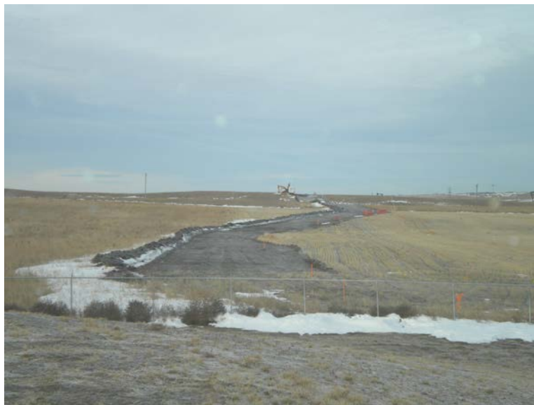
Photo 1: Looking west from Hiland Operating Plant at Project ROW, at this location pipe has been placed in the ground however topsoil has not been replaced, also ROW staking is present
