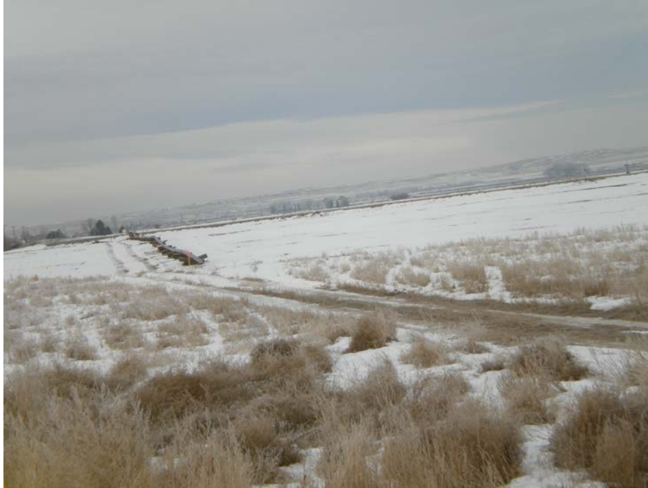
Photo 6: Looking east from 158 th Ave, ROW staking present, pipe stringing almost complete in prep for HDD of Yellowstone River.
