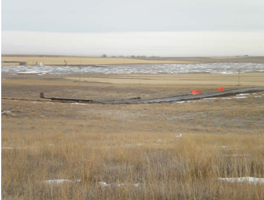
Photo 2: Looking north at ROW from County Rd 16 at 1 st drainage way crossing, not presence of silt fence on the north side of the ROW and the orange safety fence to mark the location of other pipelines crossing the construction ROW. The pipe has been placed in the ground at this location.
