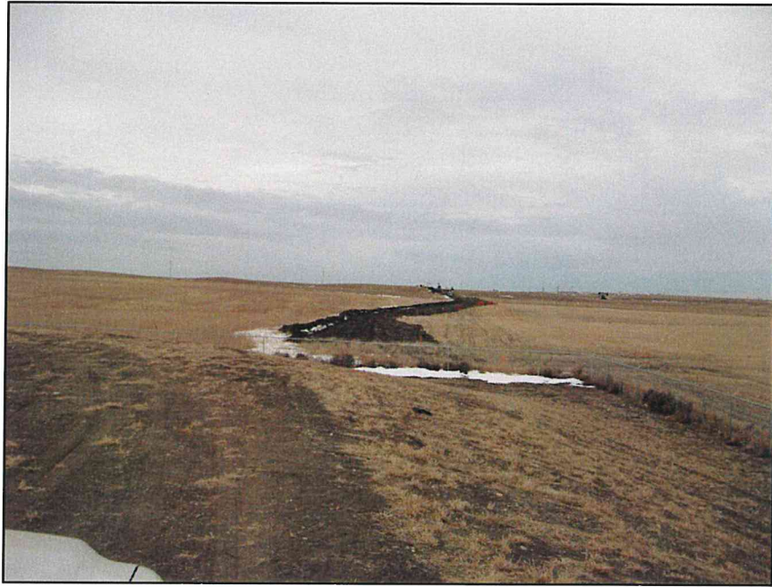
Photo 1. Taken facing west from the Hiland Operating Gas Plant. The Project pipeline crosses a wheat stubble field. The Hiland Operating 6-Inch Natural Gas Liquids pipeline (PU-12-554) project is in construction within the same ROW approximately 25' north of the existing pipeline.
