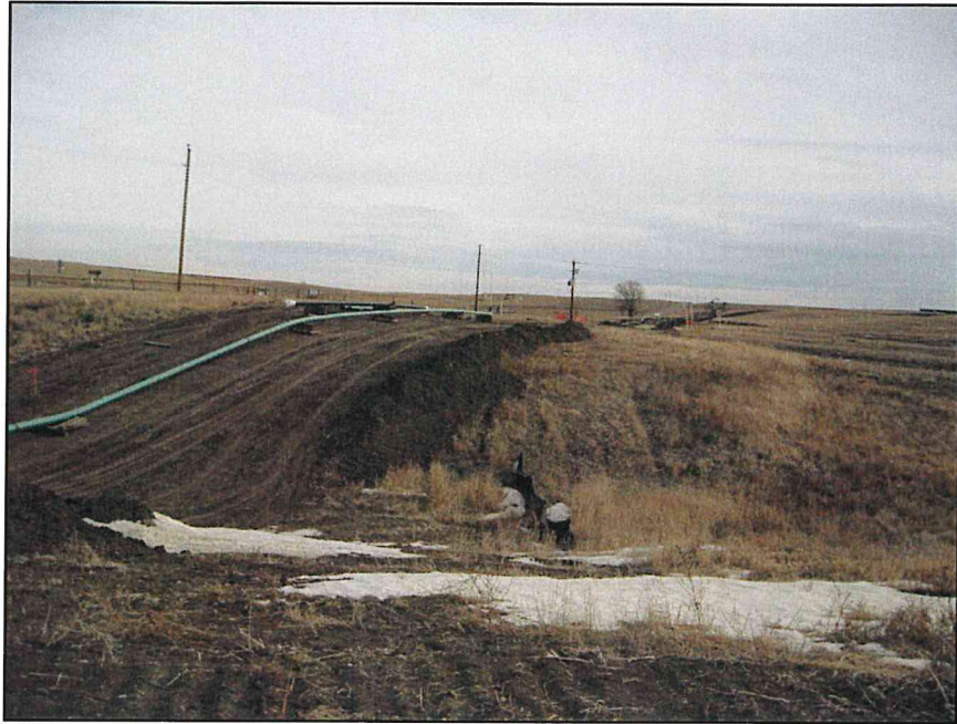
Photo 5. Taken facing east at the confluence of the main pipeline and the lateral pipeline in the northwest quarter of Section 4.
