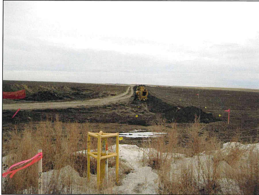
Photo 3. Taken on the eastern side of Section 2 facing east. The ROW crosses a plowed agriculture field. The Project pipeline is located beneath the topsoil windrow from the PU-12-554 project.
