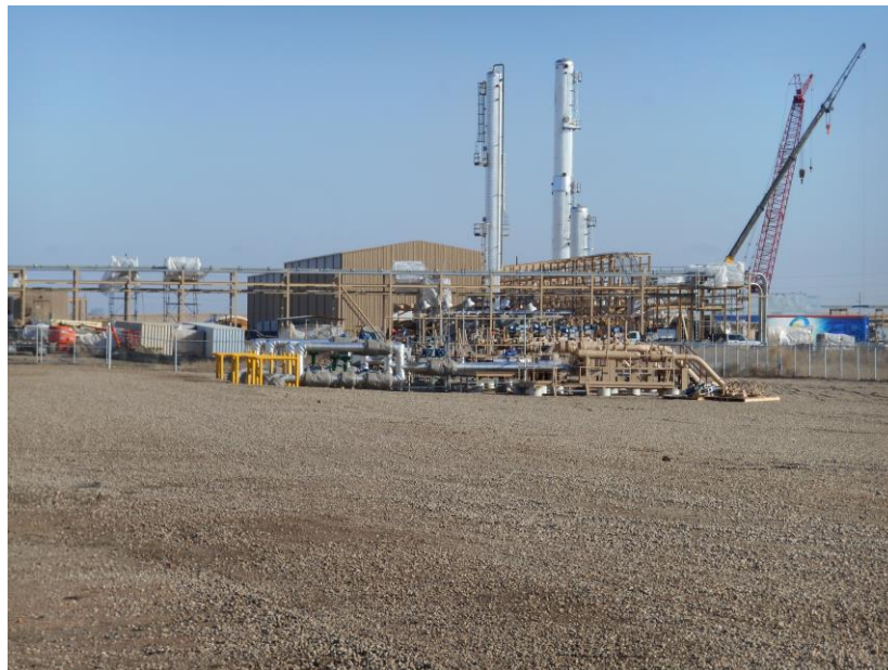
Picture 2 Inlet Gas Piping
