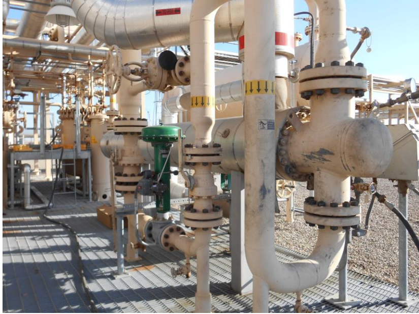
Picture 5 Heat Exchanger
