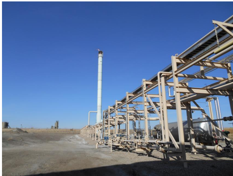
Picture 12 Flare Stack and Associated Pipe Rack
