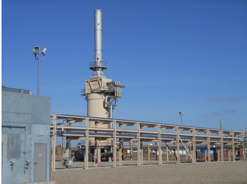
Picture 17 Hot Oil Heater
