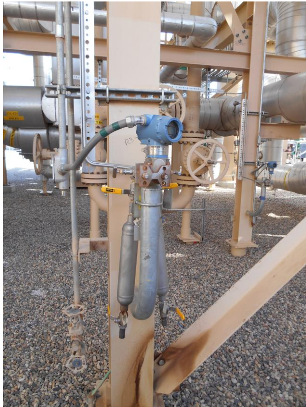
Picture 8 Blow down/ Sampling Station
