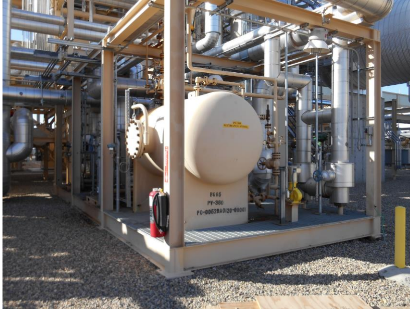
Picture 15 Methanol Vessel
