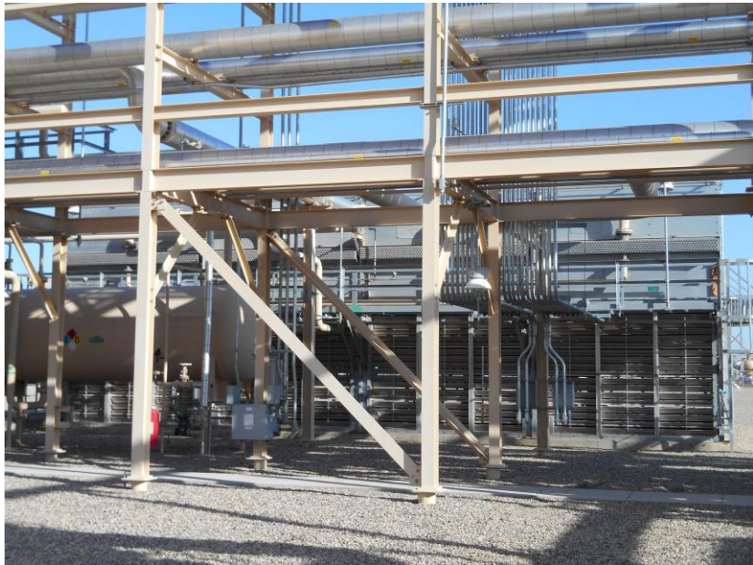
Picture 6 Propane Refrigeration Condensers
