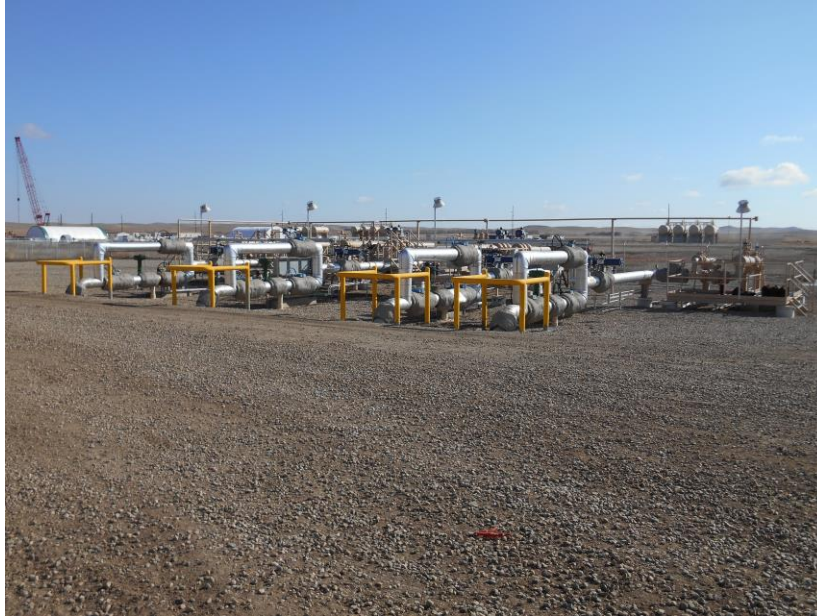
Picture 19 Pipeline Pig Receivers
