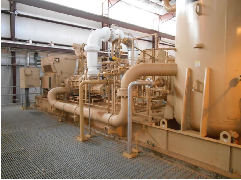
Picture 7 Propane Refrigeration Compressor
