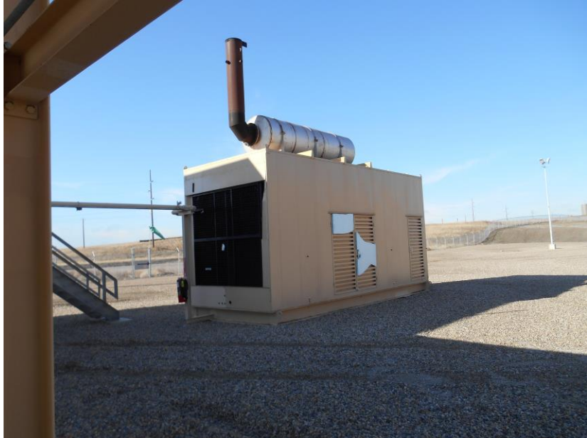
Picture 9 Diesel-Fired Emergency Electric Generator
