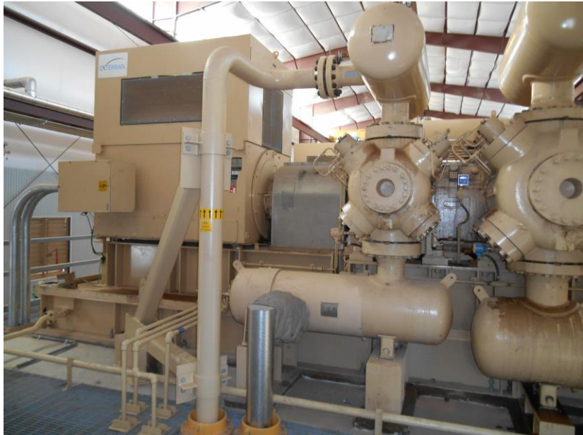
Picture 10 Residue Gas Compressor
