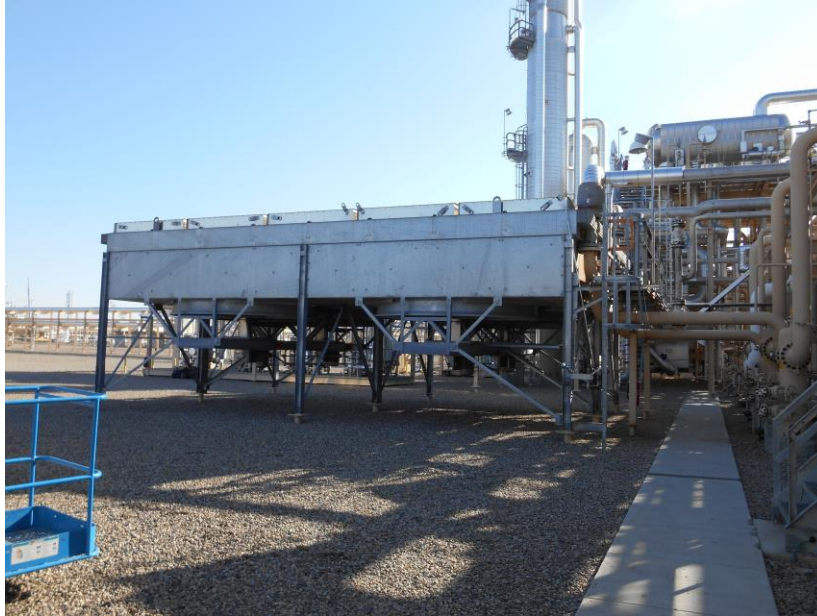
Picture 13 Residue Gas Cooler
