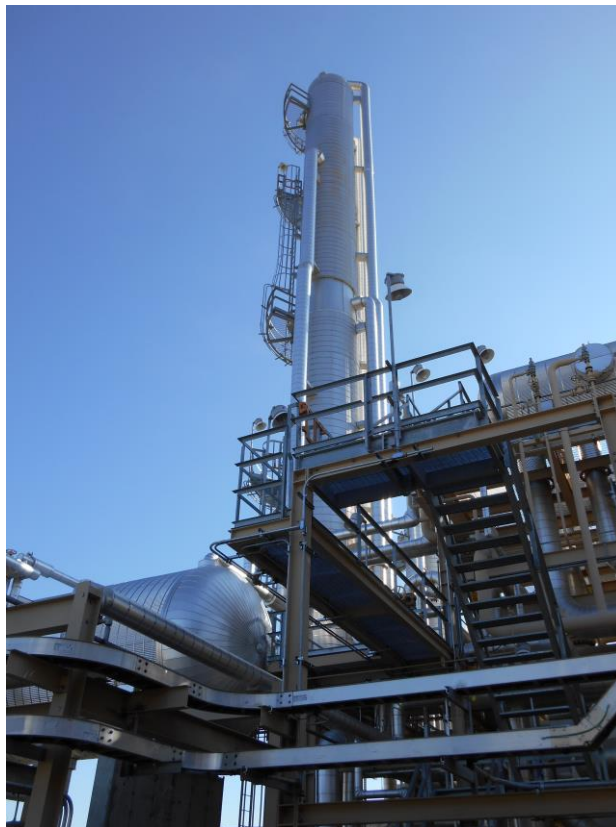
Picture 14 Fractionation Column
