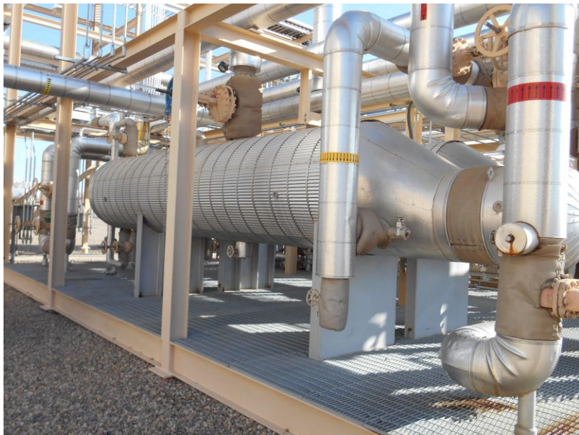
Picture 4 Stabilizer Reboiler
