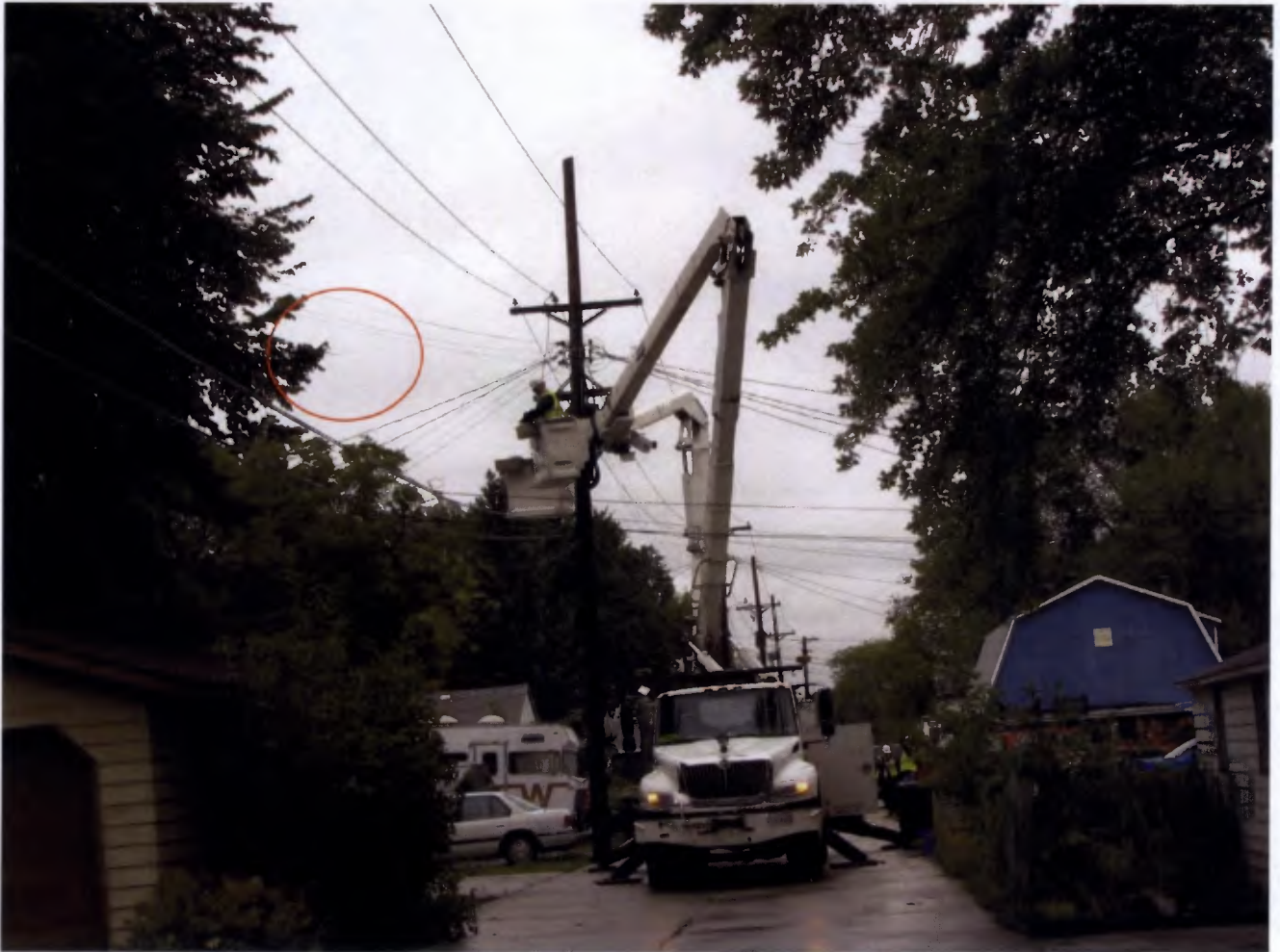
Picture was taken from the south end of the alley between 7 th and 8 th streets, looking to the north. Crews are working near the T53 transformer. The contacting tree branch on the west side of the alley is slightly visible (see red circle) below the secondary wires.
