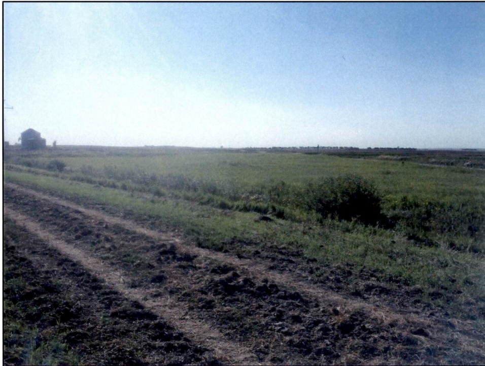
Photo 2. Station 288+00 Looking southeast at a roadways that had been horizontally directionally drilled.
