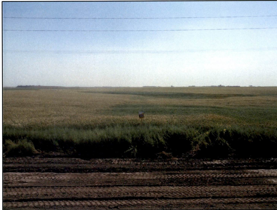
Photo 9. Station 146+00 Looking east at settlement of the pipeline trench in a wheat field.
