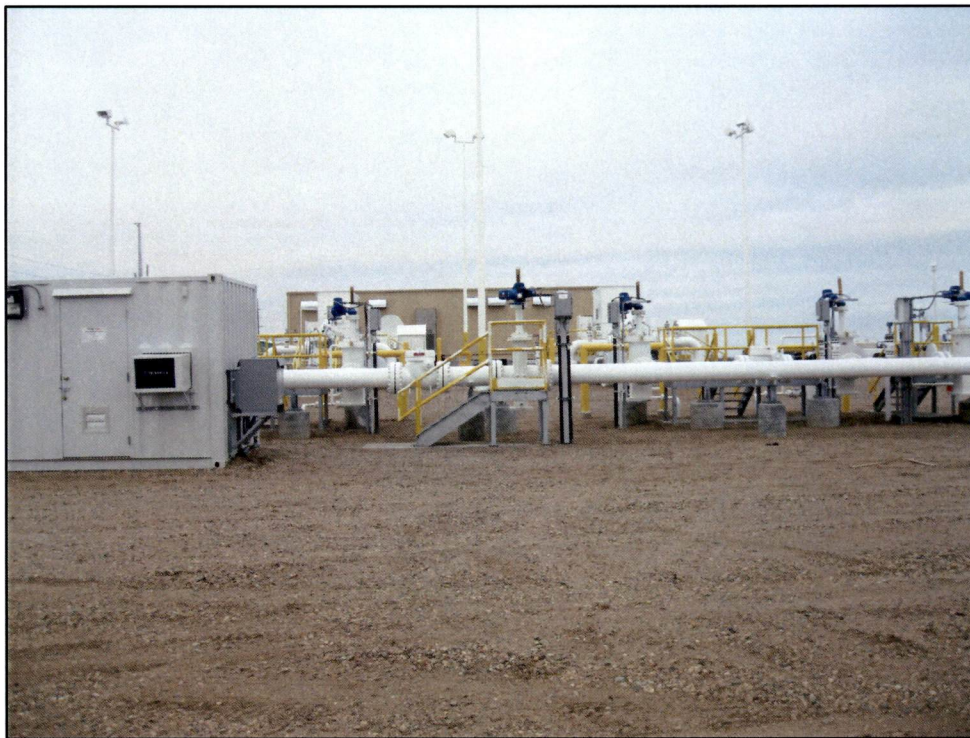
Photo 16. Kenaston Pump Station pumps, meters, and piping.
