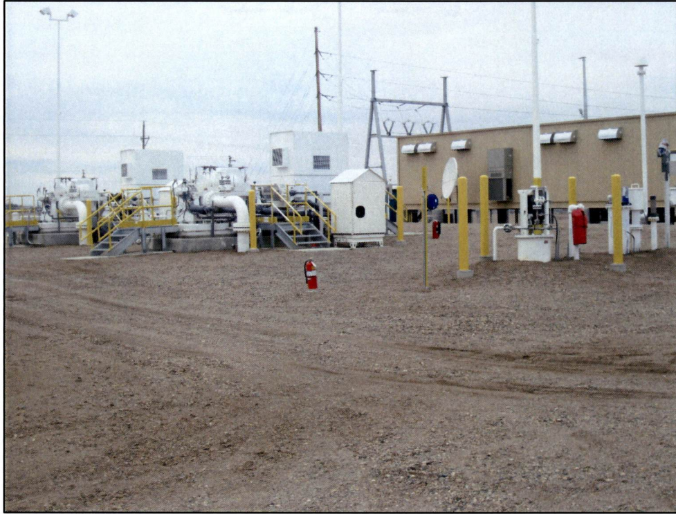
Photo 17. Kenaston Pump Station pumps, meters, and piping.
