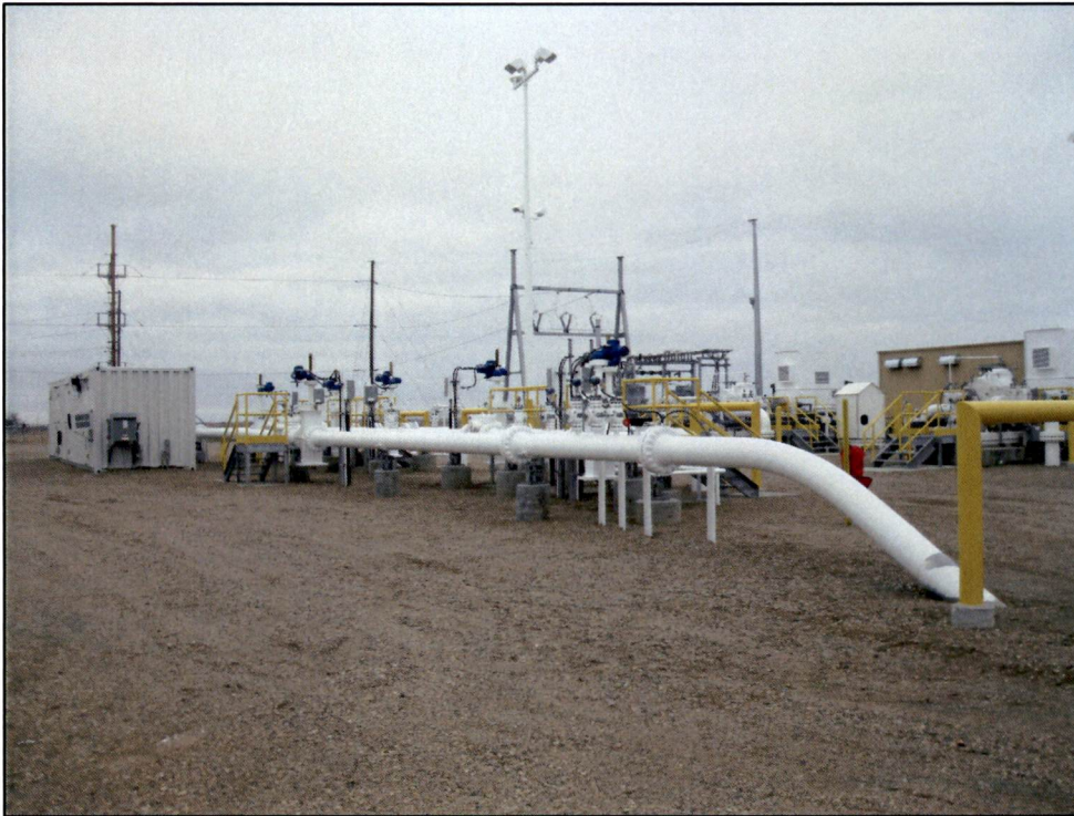
Photo 12. Lignite Pump Station.
