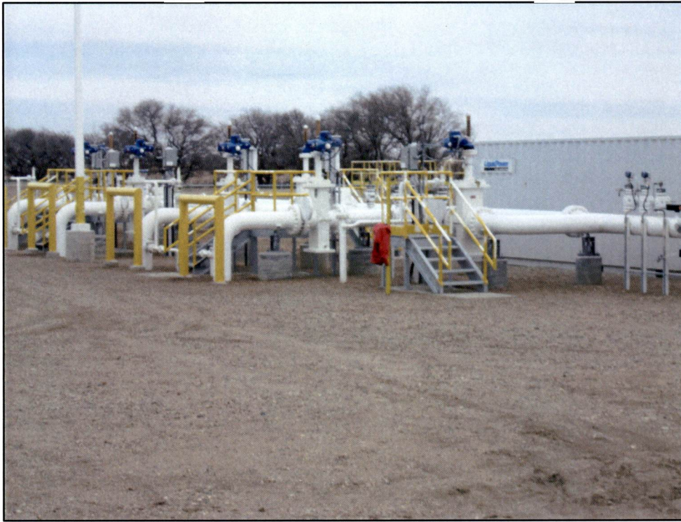
Photo 15. Kenaston Pump Station above ground piping.
