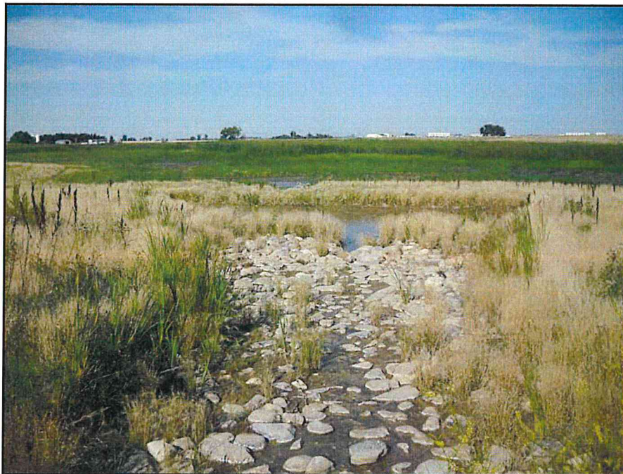
Photograph 6. A storm water drain from the BTUL flows into a retention pond before the mitigation wetland. Excessive runoff caused water to flow out of the retention pond and erode the upland buffer.
