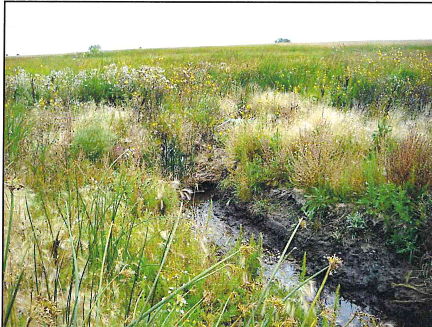
Photograph 9. Close-up of erosion cut located at the end of the stormwater drain.
