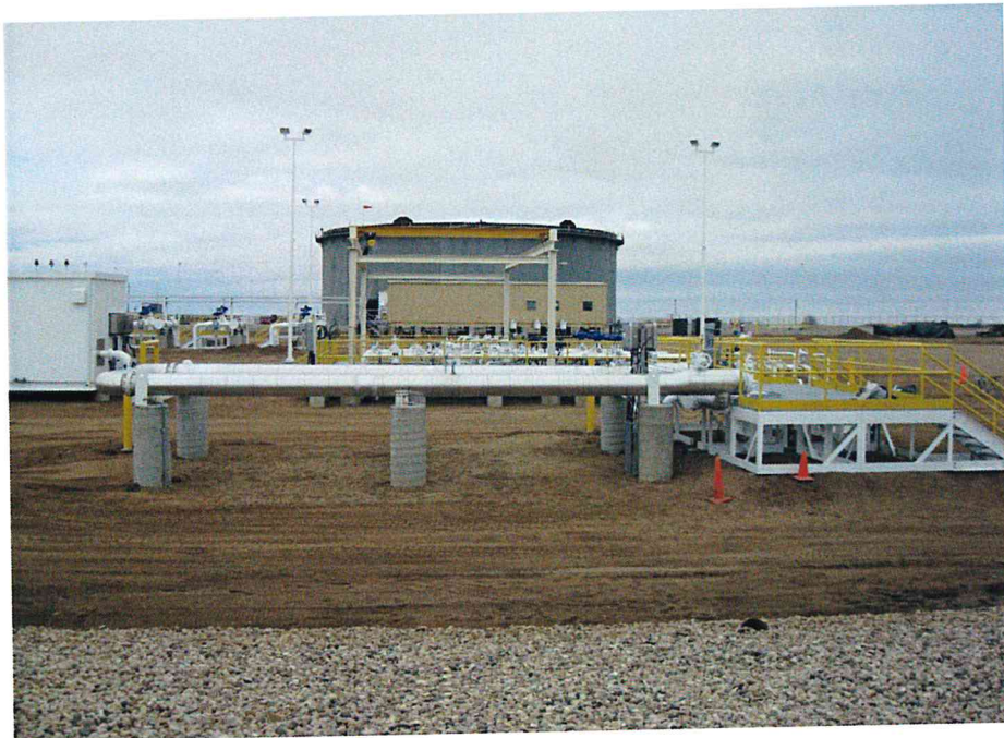
Figure 12: Pumps & Meters at Berthold Pump Station
