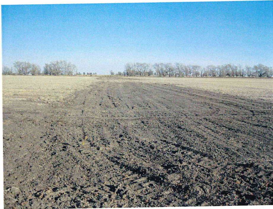
Figure 4: STA 1140+15 Looking East at Pipeline Trench Area that was graded in October/November 2013 (between M.P. 55.7 – 54.8)
