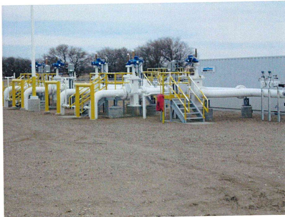
Figure 24: Pumps & Meters at Kenaston Pump Station
