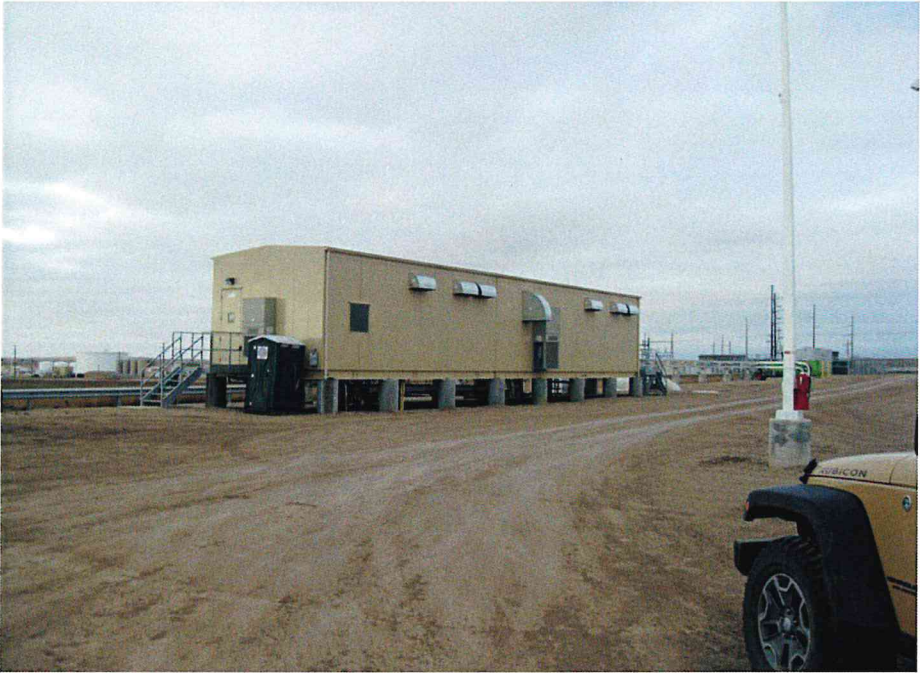
Figure 16: Electrical Equipment Building at Stanley Pump Station
