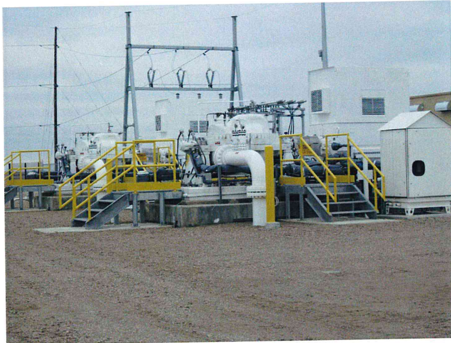
Figure 23: Pumps & Meters at Lignite Pump Station
