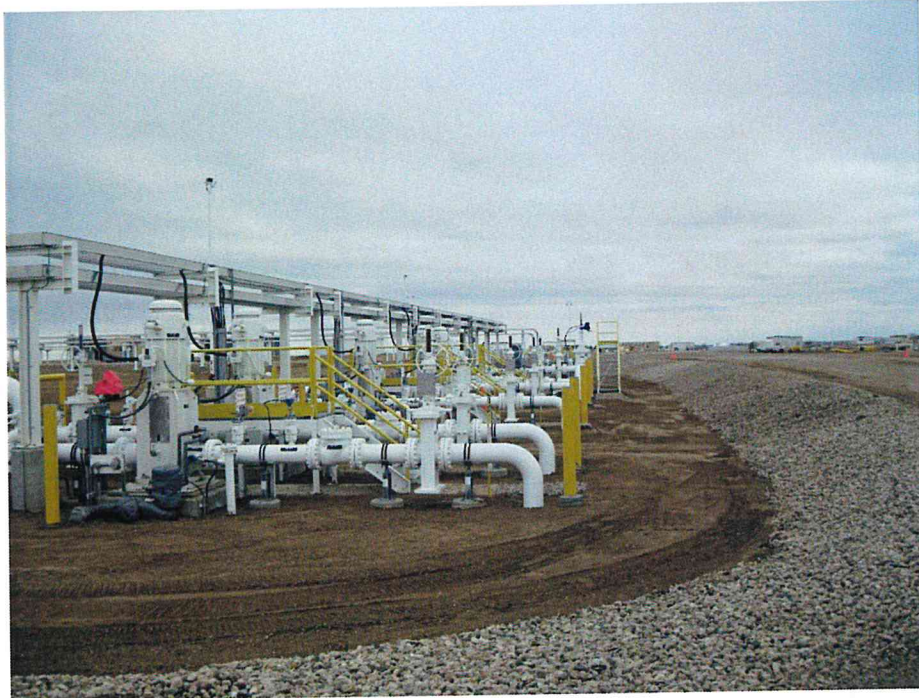
Figure 13: Pumps & Meters at Berthold Pump Station
