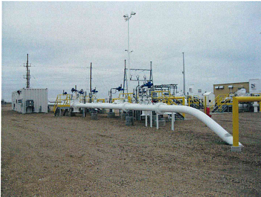
Figure 22: Pumps & Meters at Lignite Pump Station
