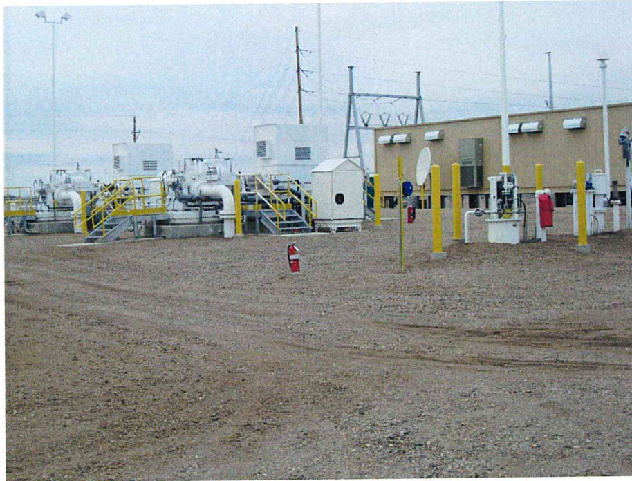
Figure 25: Pumps & Meters at Kenaston Pump Station
