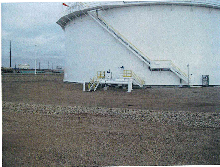
Figure 19: The Tank at Beaver Lodge Pump Station
