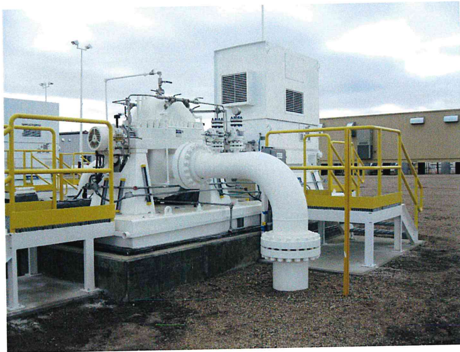
Figure 18: Pumps & Meters at Beaver Lodge Pump Station
