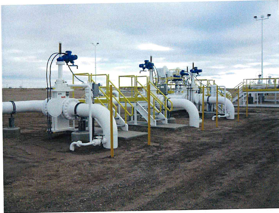
Figure 17: Pumps & Meters at Stanley Pump Station
