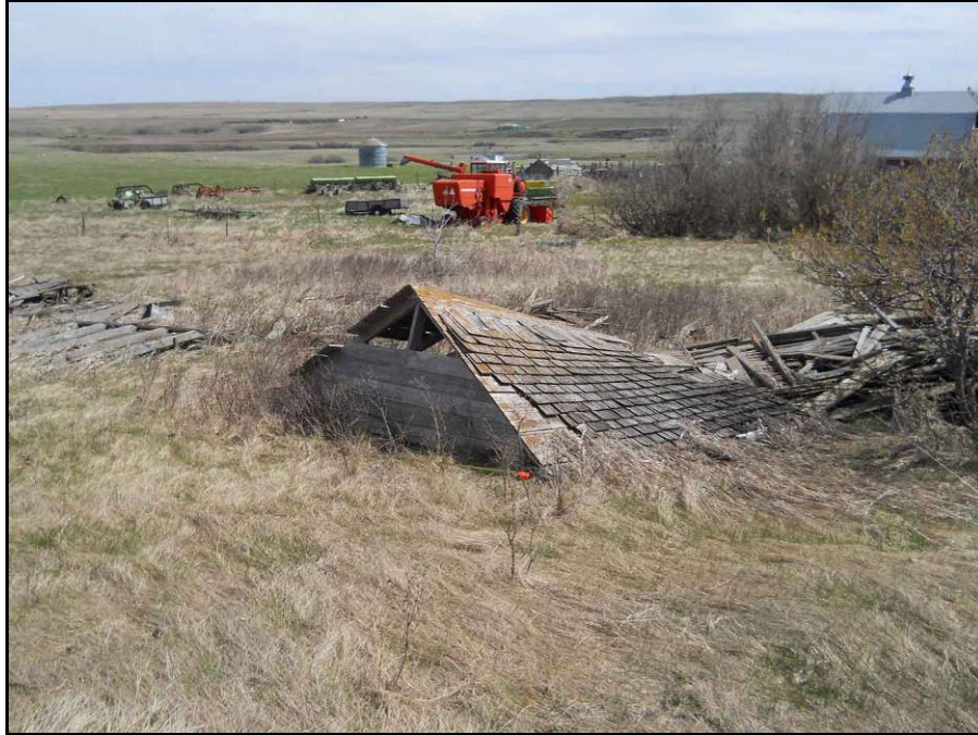
Figure 50. 32WI1154. Feature 1, dilapidated roof and gable, with tape measure set at 3 feet, facing south.
