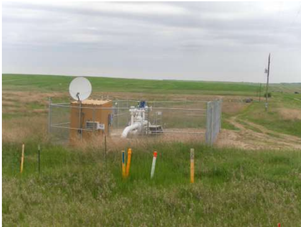
Photo 2 – Typical mainline block valve station
