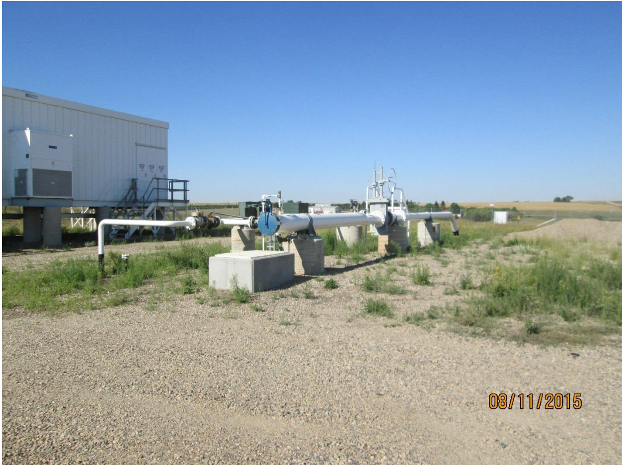
Photo 2 – Beaver Lodge Meter Station site.
