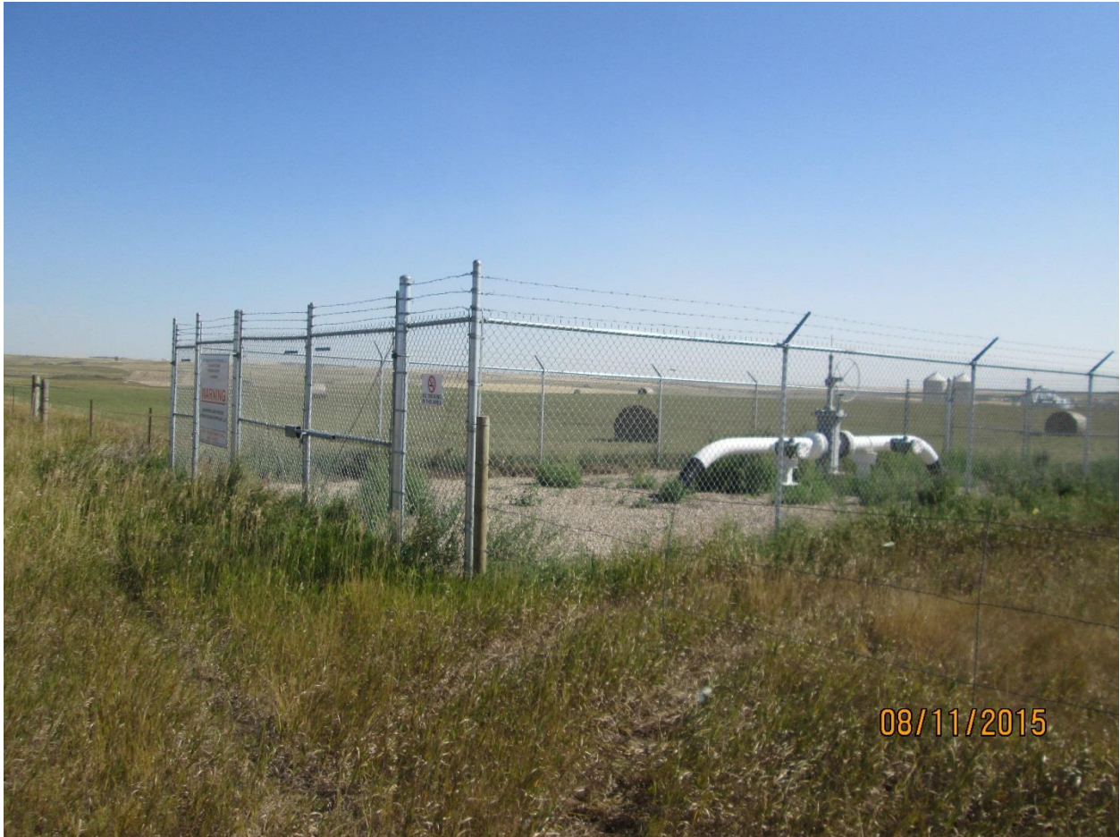
Photo 3 – Midway mainline block valve station.
