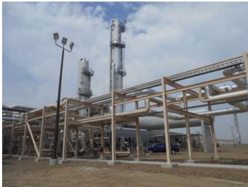
Picture 4 Pipe Racks with Fractionation column in the background
