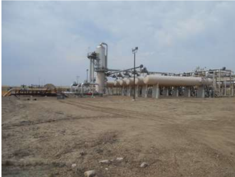
Picture 1 Inlet Gas Piping
