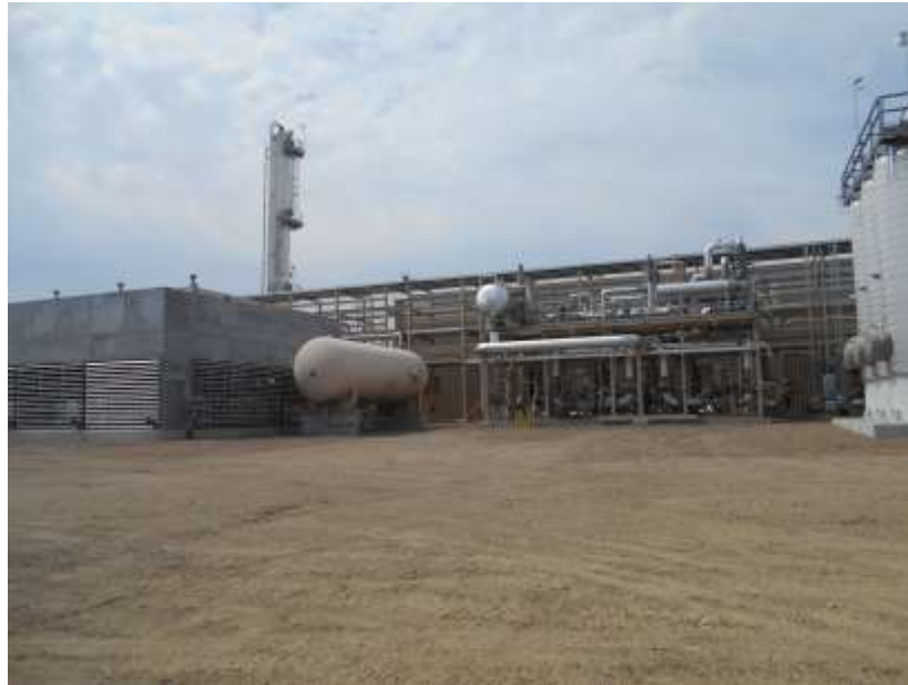
Picture 3 Pipe Racks
