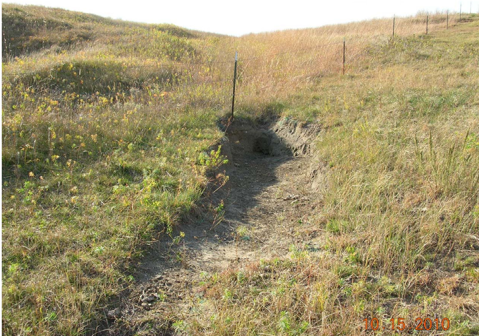
Figure 10. Erosion in a drainageway in the SE 1 / 4 of the NW 1 / 4 of the SW 1 / 4 of Section 18 (Tract 1C) at the mine disturbance boundary about 200 feet northeast of soil probe number 88.
