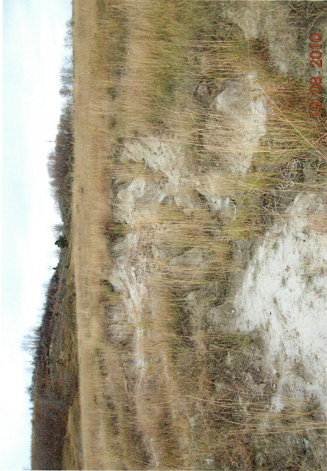
Figure 7. Erosion and piping west of Pond 1 in the N \frac{1}{2} of the NW \frac{1}{4} of Section 31 (Tract 4C) south of soil probe number 55.
