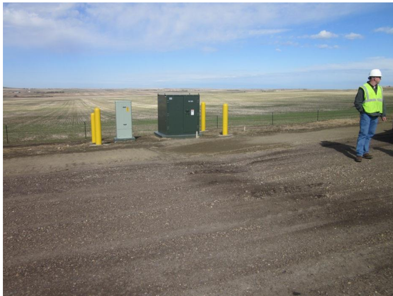
Photo 12. Direction: West. Transformer with appropriate safety bollards in place. The access road in this photo had a slight low area during the interim inspection, which had been repaired by the time of the final inspection.
