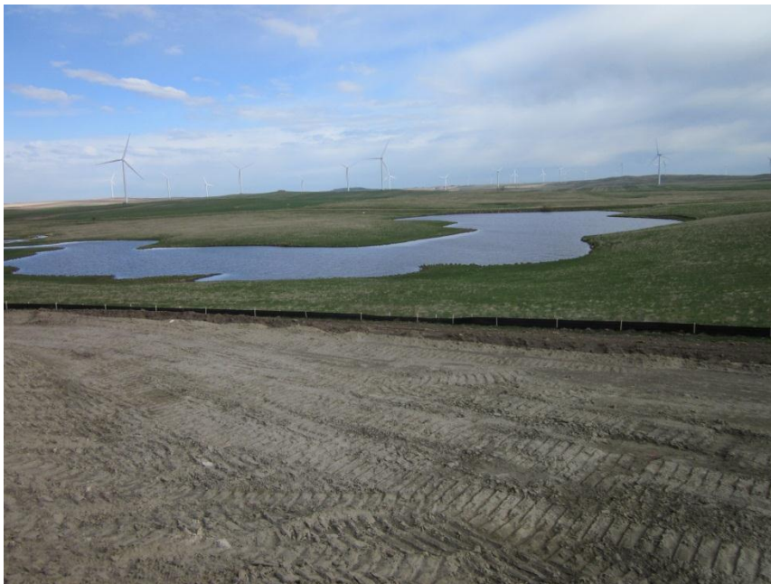
Photo 10. Direction: Northwest. Example silt fence observed during the interim inspection preventing erosion to nearby wetland at Structure 208.
