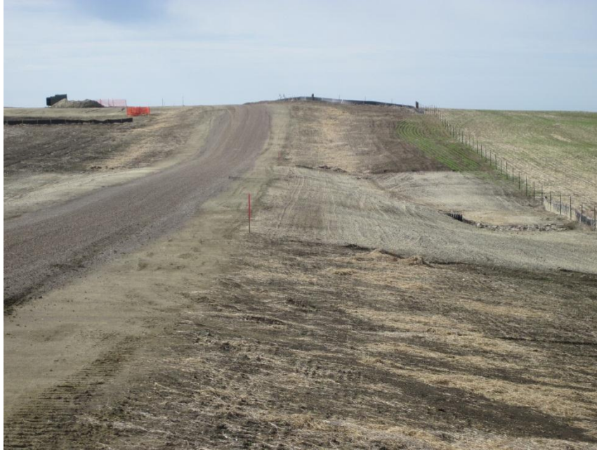
Photo 13. Direction: South. Access road to Structures 224 and 225. Note mesh netting and rocks at base of culvert for erosion control.
