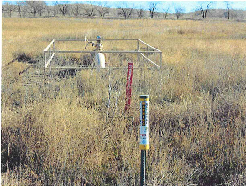
Photo 9 – Direction: East – Pipeline valve station near pipeline mile marker 6.5. McKenzie County Road 36 road crossing. Notice pipeline markers.
