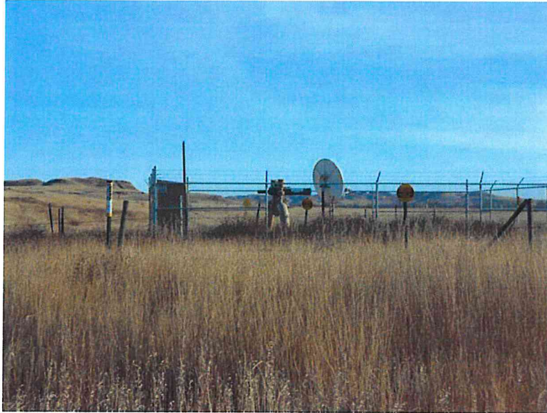
Photo 25 – Direction: Southeast – Pipeline valve station near pipeline mile marker 44. ND 16 Highway crossing.
