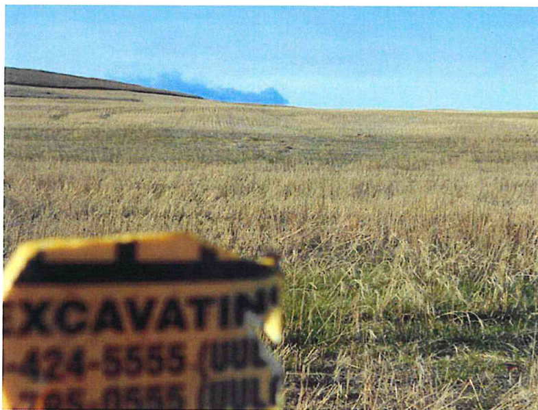
Photo 18 – Direction: West – Showing revegetation near pipeline mile marker 18.5. Notice damaged pipeline marker.
