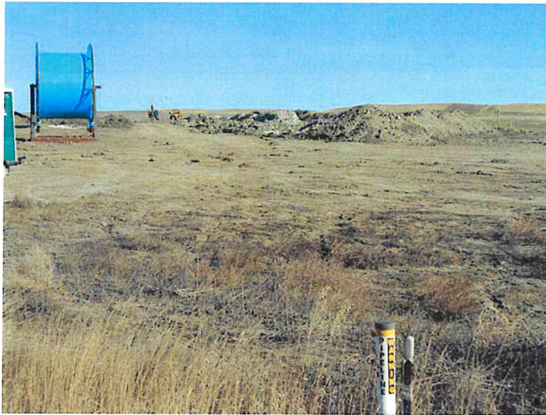
Photo 19 – Direction: East – Showing revegetation near pipeline mile marker 20.5. McKenzie County Road 27 road crossing. Notice new pipeline being installed adjacent to this pipeline.
