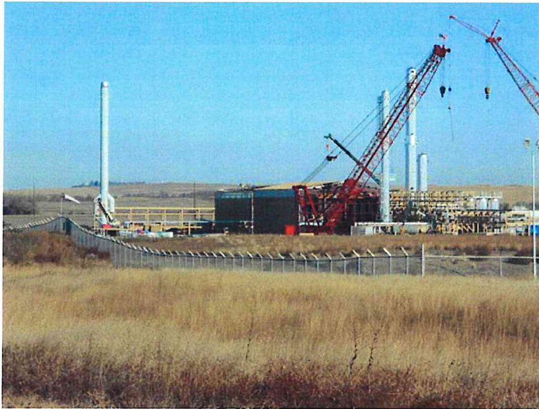
Photo 1 – Direction: North – Garden Creek Gas Plant
