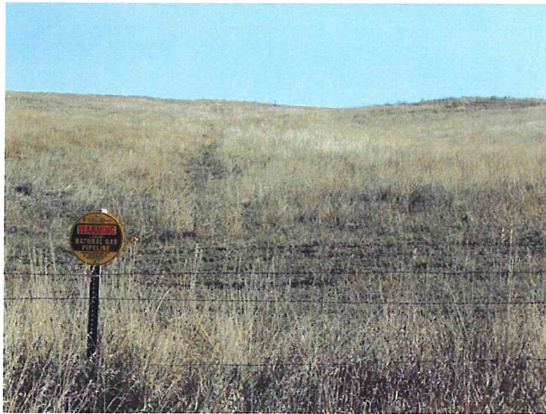
Photo 5 – Direction: East – Showing revegetation at McKenzie County Road 36 crossing near pipeline mile marker 4.
