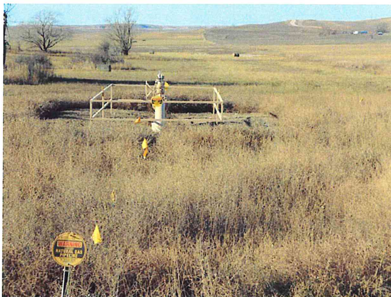
Photo 10 – Direction: West – Pipeline valve station near pipeline mile marker 6.5. McKenzie County Road 36 road crossing. Notice pipeline markers.
