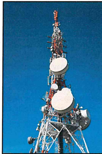
Figure 1: Mast with terrestrial microwave antennae
