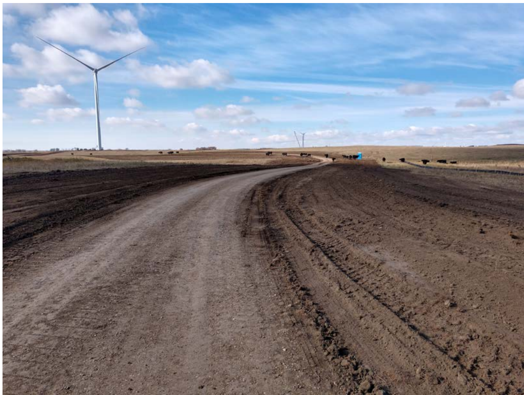
Photo 6. Taken facing southwest along access road to Turbine 42. Road side slopes have been graded to final contours.
