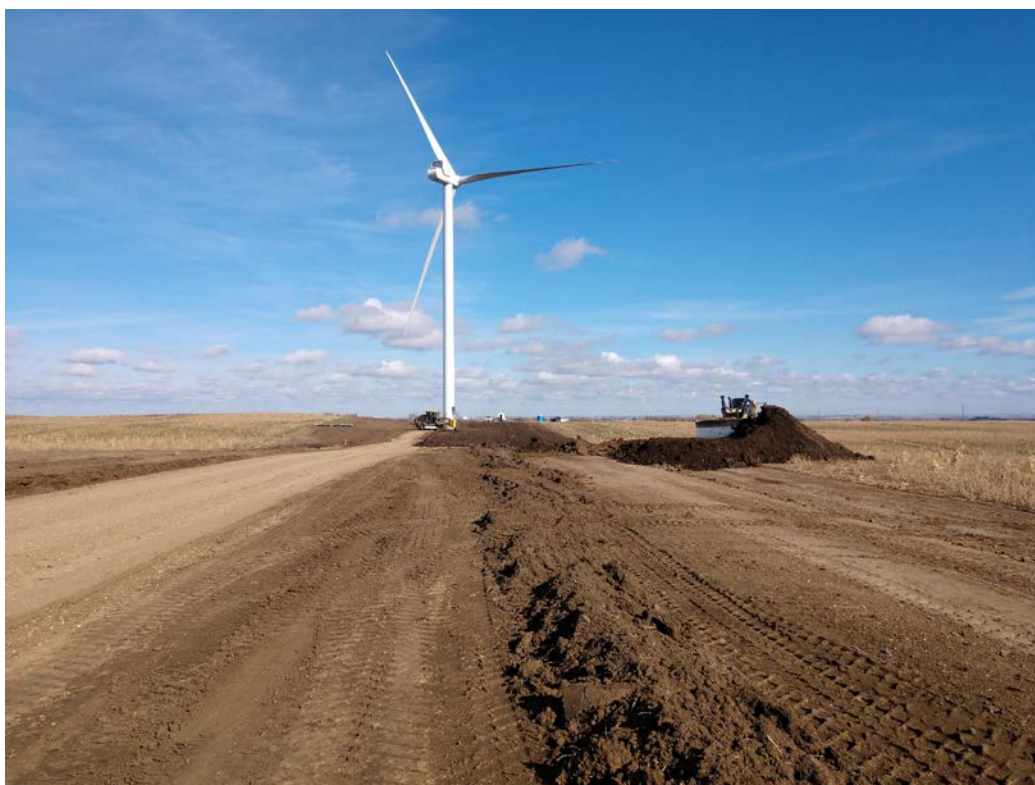
Photo 8. Photo taken facing north along access road to Turbine 64. Earthwork has commenced to redistribute topsoil along access road.
