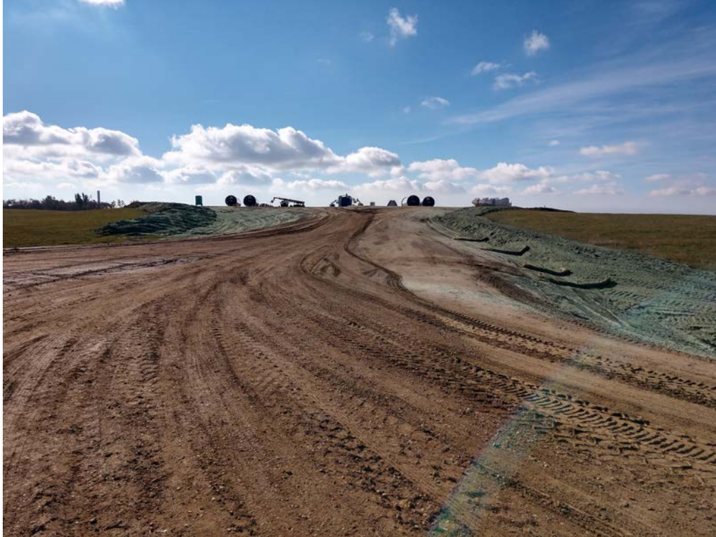
Photo 5. Photo of Turbine 54 access road. Hydromulch has been applied to topsoil to stabilize soil prior to freezing weather. Photo taken facing south.
