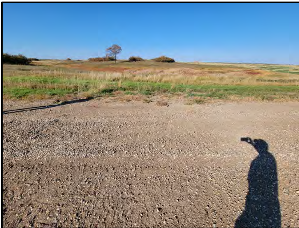
Photograph 5. View looking west from the access road intersection to Turbine 14. Surface water flow has caused rock to wash into the road shoulder. Crews are aware of this and working towards remediation.
