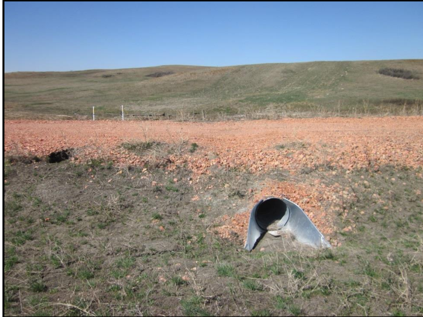
Photo 2. Direction: West. Access road (north-south alignment) crossed by the pipeline route. The as-built indicated the pipeline was bored underneath what was previously a trail through a field. The road had recently been built up and surfaced with scoria as access to new oil wells to the south. The road had a shallow dip where the culvert had been installed and the soil had settled. The Hiland representative stated that an oil company built and was responsible for the condition of the access road.
