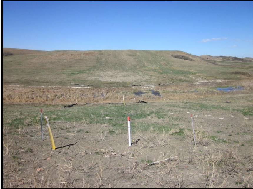
Photo 3. Direction: West. Crossing of Dry Creek on the east end of the pipeline route. Pipeline markers and cathodic protection system markers were in place. Note the new fence installed parallel to the creek in the foreground. The pipeline route is visible on the far side of Dry Creek going upslope to rolling hills of native prairie in the NE \frac{1}{4} of Section 19. Note the bare patches of soil where vegetation had not yet established.
