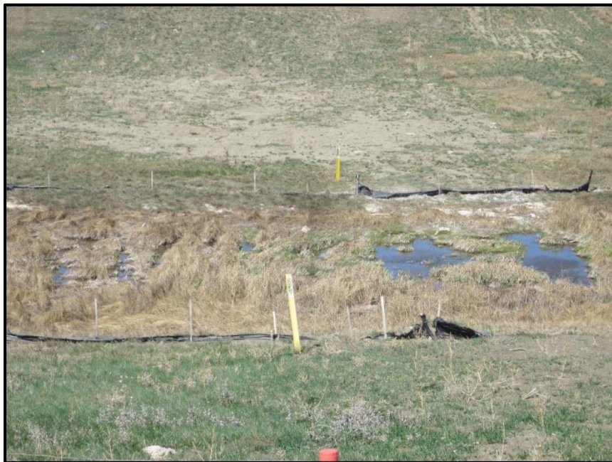
Photo 4. Direction: West. Closer view of Dry Creek crossing with silt fences on both sides. The vegetation and lowest margins of Dry Creek did not appear disturbed, which confirmed that the creek was bored underneath. Arrow had planned an 80-foot vegetation buffer on either side; however, the soils within the corridor were obviously disturbed up to within a few feet of the edge of the creek.
