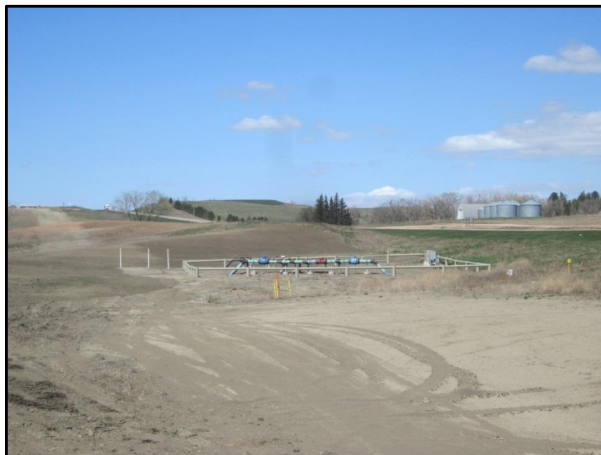
Photo 10. Direction: West. West end of pipeline at the tie-in to the existing 4 Bears Pipeline in the NE \frac{1}{4} of the NE \frac{1}{4} of Section 24.
