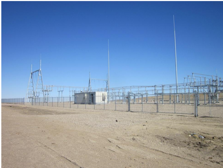
Photo 34. Direction: Northeast. Merricourt substation showing storm water control culverts and approaches. Substation appeared to be in good order with no erosion or other impacts noted.
