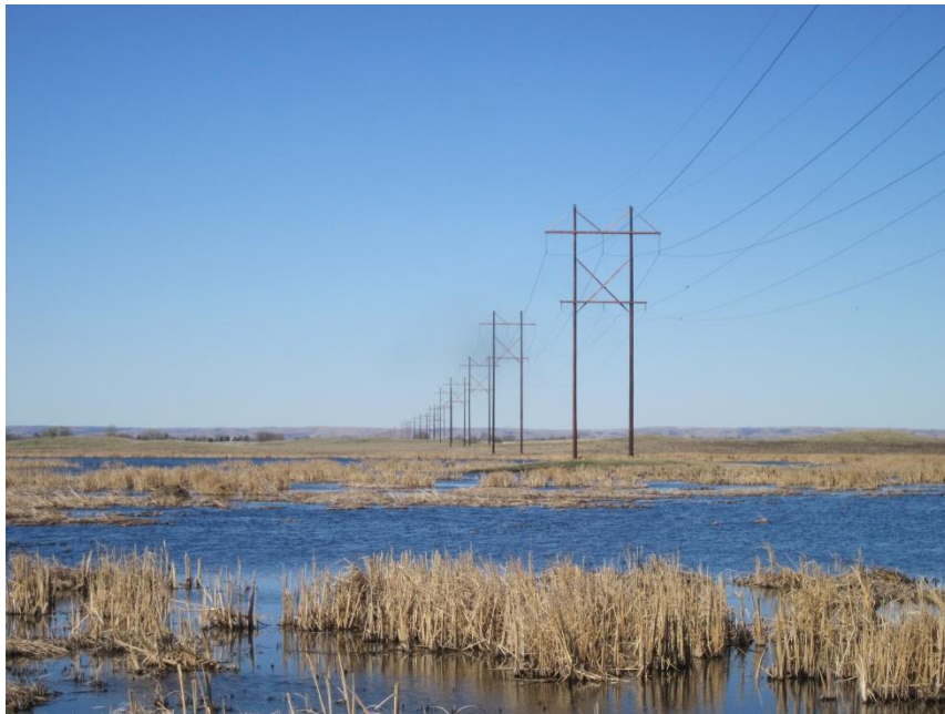
Photo 8. Direction: West. This is a closer picture of the wetland crossing shown in Photo 8. Note structure is not located in wetland, but on small island.
