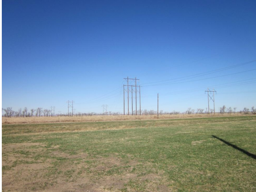
Photo 5. Direction: Northwest. New line leaving the Ellendale substation, which is located just behind where this photo was taken. Notice new line (larger structure on the left) parallels an existing line out of the substation.
