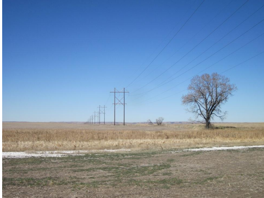
Photo 13. Direction: West. Transmission line spanning a cattail slough approximately 8 miles west of the Ellendale substation.
