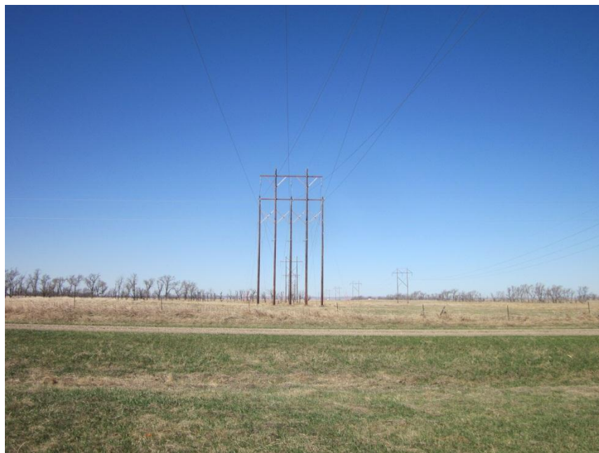
Photo 6. Direction: West. Double circuit transmission line leaving substation traveling west.
