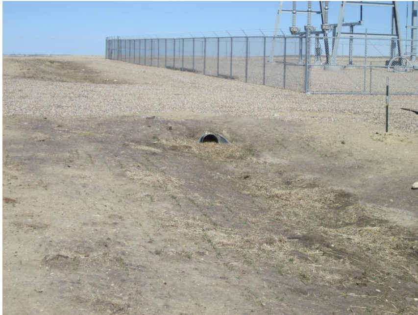
Photo 33. Direction: North. Example of storm water and erosion control measures with culvert underneath access road to substation.
