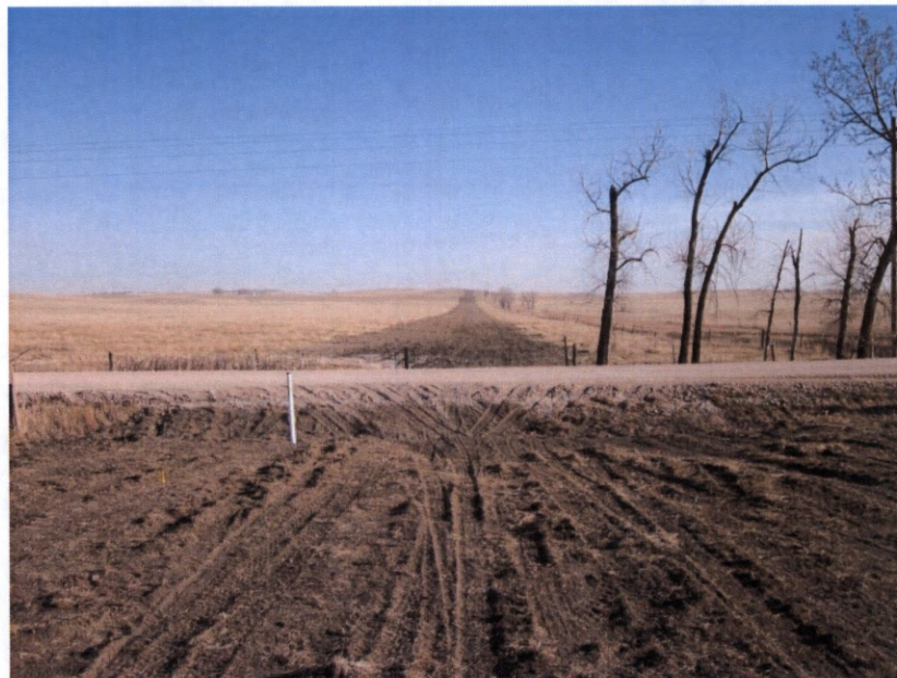
Photo 4. Direction: North. This photo shows the right-of-way of the Whiting Pipeline where it bores under 32 nd Street.
