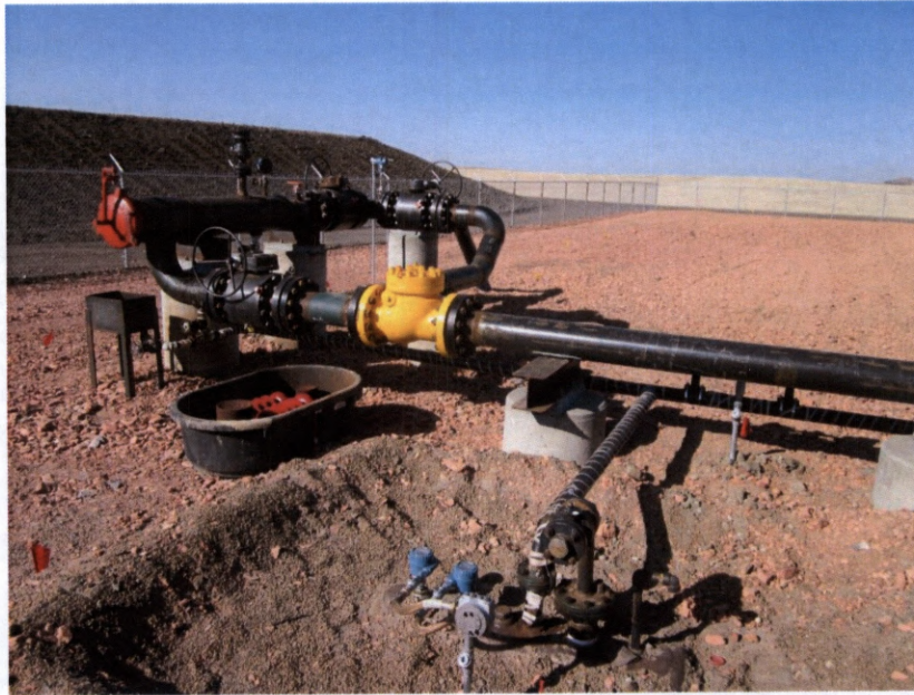
Photo 23. Direction: Southwest. Skunk Hill receiver indicating the end of the pipeline right-of-way; no erosion or settling was noted at receiver. Pad was in good order with appropriate safety measures in place. Located in Section 21 of Township 141N Range 98W.
