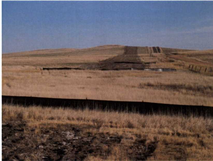
Photo 9. Direction: North. This is a closer picture of the pipeline boring underneath a wetland. Note erosion control structures in place.
