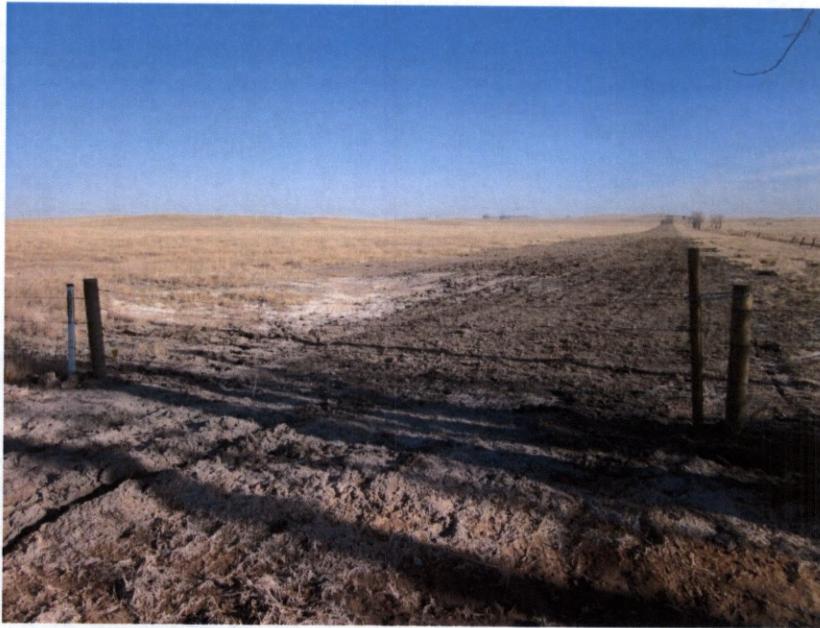
Photo 5. Direction: Northwest. Northern side of 32 nd Street bore. Fence had been repaired and was in good condition. No erosion or other problems were evident.
