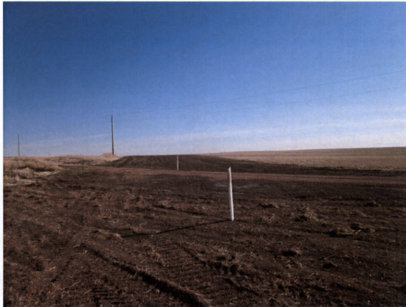
Photo 19. Direction: Northeast. This photo shows the right-of-way of the Whiting Pipeline where it bores under 124 th Avenue at observation point 136 ( Figure 1 ). Note signage on both sides of the road, which was typical of all road crossings along the pipeline route.
