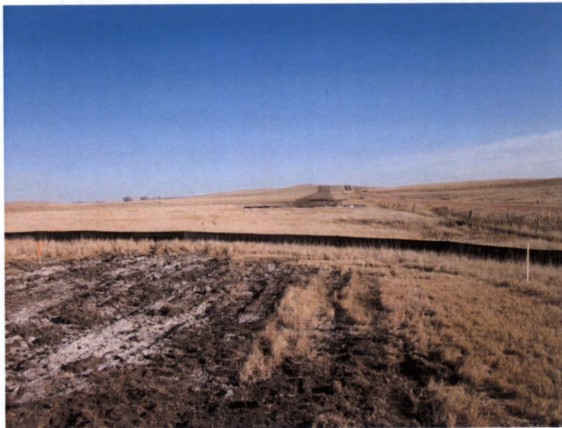
Photo 8. Direction: North. Photo shows pipeline right-of-way where it bores underneath a wetland at observation point 127 ( Figure 1 ). Erosion control structures were in place and no erosion to the water body was evident.
