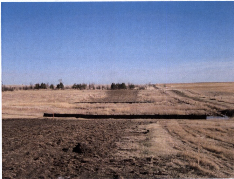
Photo 12. Direction: North. Photo shows pipeline right-of-way where it bores underneath a wetland at observation point 131 ( Figure 1 ). Erosion control structures were in place and no erosion to the water body was evident. Tree row in background was also bored with no impacts to surrounding vegetation.
