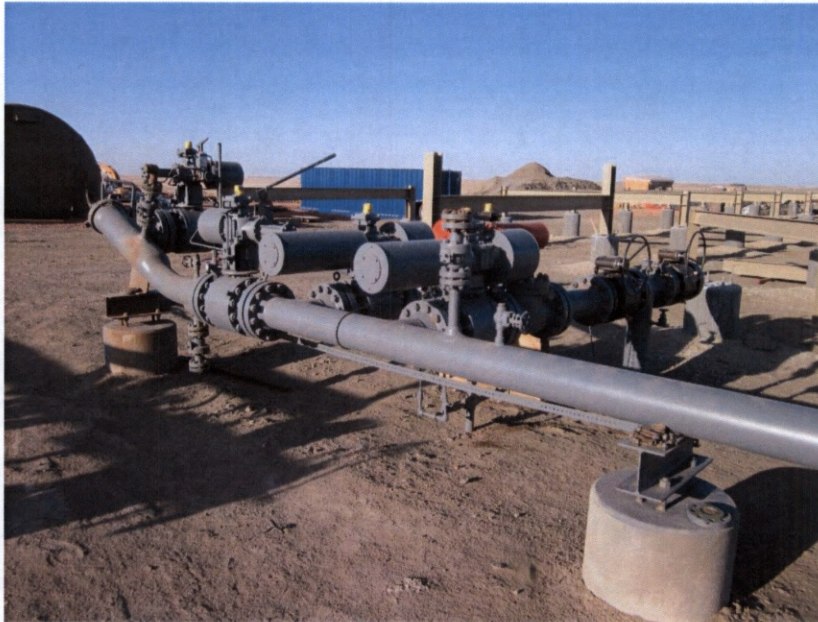
Photo 1. Direction: Southwest. Start of pipeline at Belfield Oil Terminal. All aboveground structures were in order and constructed per PSC and application guidelines. Located in Section 14 Township 141N Range 99W.
