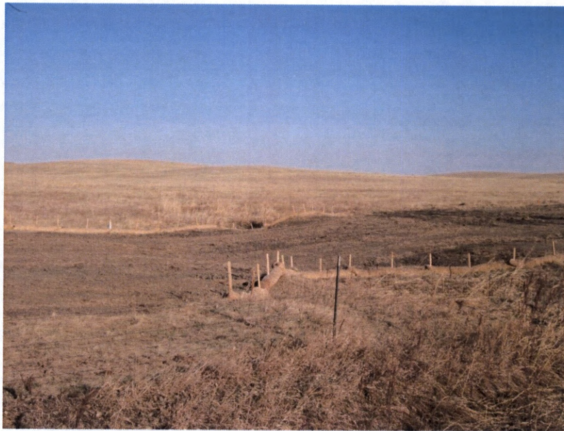
Photo 6. Direction: West. Photo shows erosion control structure located at a low area along the pipeline right-of-way at observation point 125 ( Figure 1 ). Structures similar to this were located at all low areas and wetlands throughout the right-of-way.
