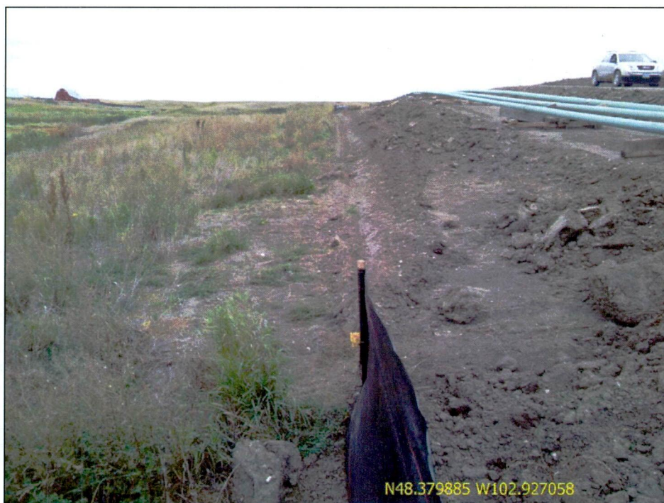
Figure 8. Additional silt fencing recommended to be installed along downslope of ROW just east of Highway 40 crossing.
