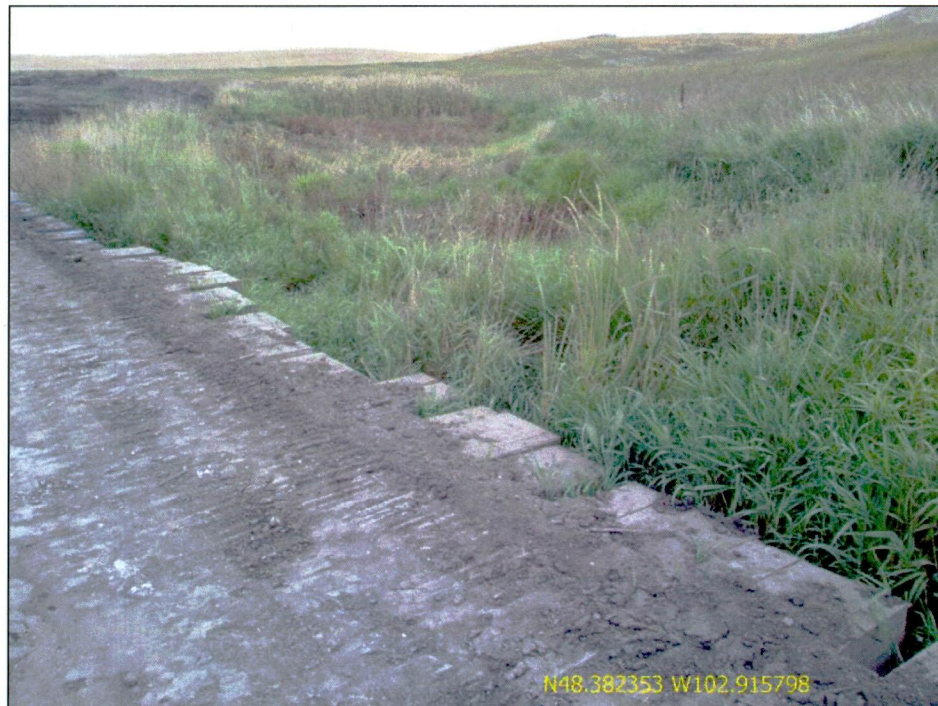
Figure 4. Wooden mats are in place for equipment to traverse the stream/wetland area. Additional silt fence or other ECD was recommended at both ends of crossing to reduce chance of sediment migration.
