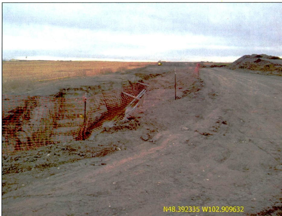
Figure 1. Photo taken of ROW looking south from 67 th Street NW. The HDD bore pit work area and foreign line crossing is visible.
