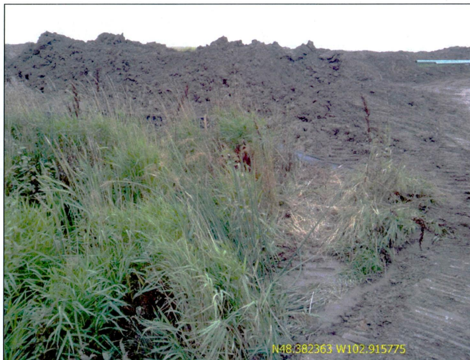
Figure 5. Silt fencing damaged by construction equipment from recent HDD pit digging which was in need of maintenance. Hess EHS Advisor assured maintenance will occur immediately.
