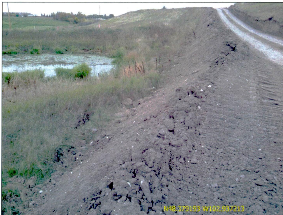
Figure 10. Photo of temporary access road built up along the edge of a wetland complex. Additional ECDs recommended to reduce potential sediment deposition into wetland.
