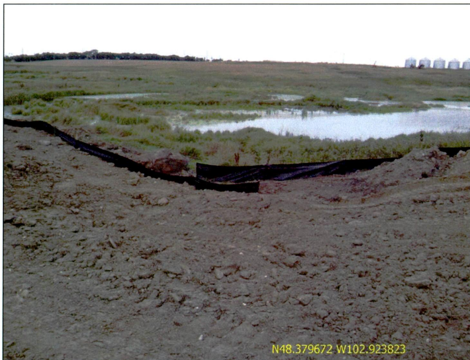
Figure 7. Silt fence improperly installed directly above stream/wetland complex. No sediments had washed through. Hess EHS Advisor assured maintenance will occur immediately.
