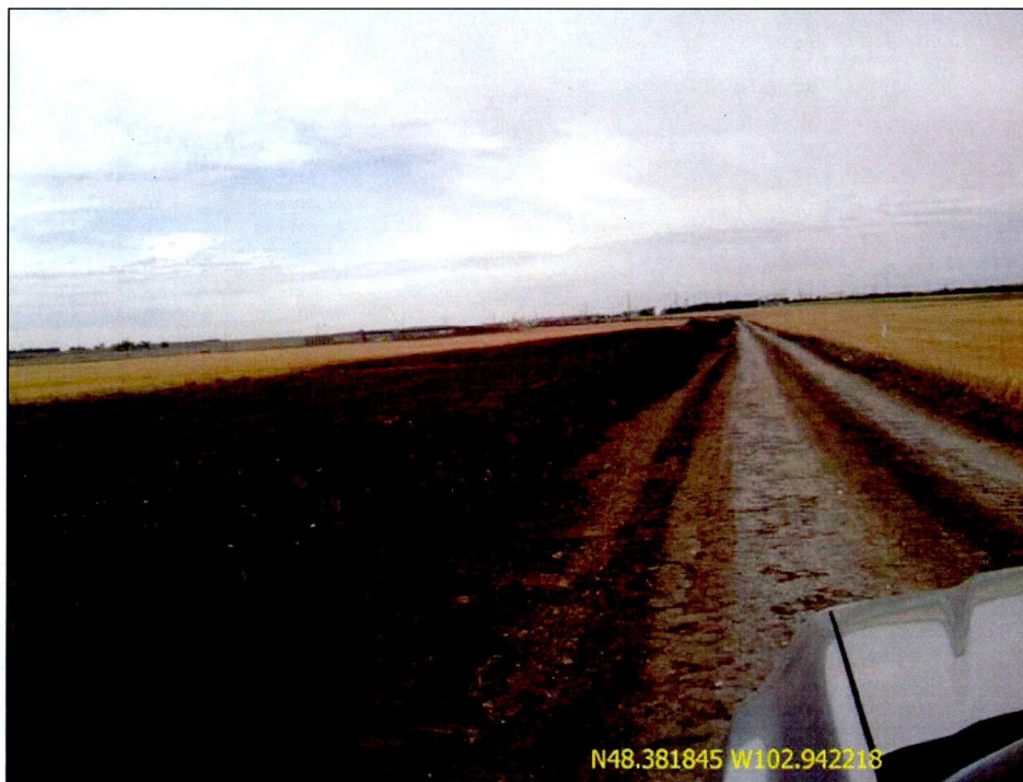
Figure 11. Photo of ROW in which pipeline installation has occurred and topsoil has been redistributed across ROW (except for on utilized access route).
