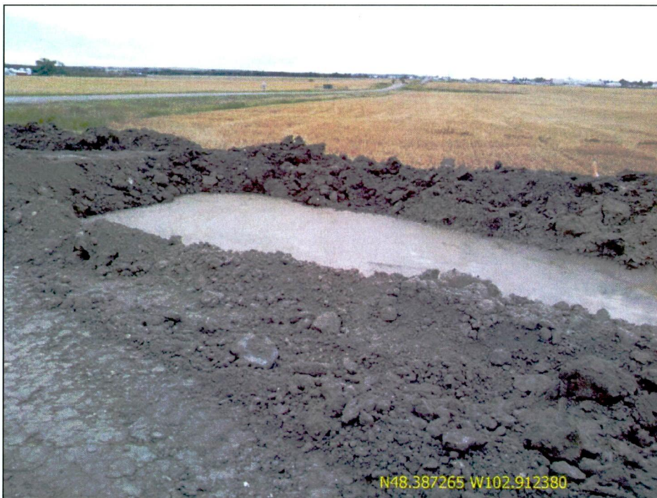
Figure 2. Photo of dewatering pit constructed of trench sub-soils within the ROW. These temporary sediment catchments will be reclaimed as HDD bore is complete and pits are backfilled.
