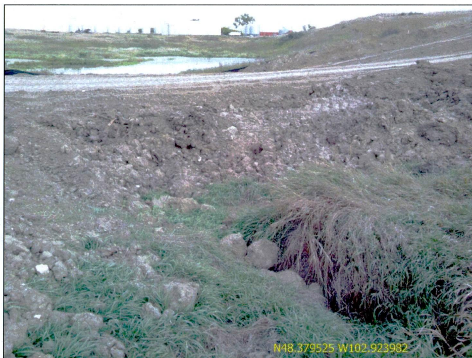
Figure 6. Photo of ephemeral drainage crossing. Steel drain pipe is in place; however, the entrance was covered with soil and may have prevented proper drainage.
