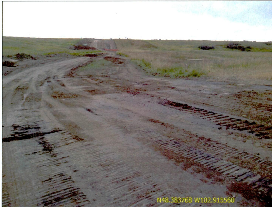
Figure 3. Photo of first stream crossing south of 67 th Street NW. ROW width has been reduced and HDD bore has taken place.
