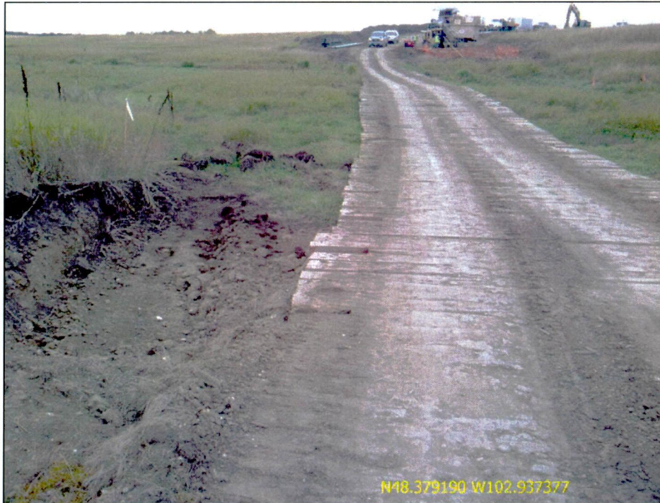
Figure 9. Photo of wooden matting placed to minimize surface impact of stream/wetland crossing west of Highway 40. Additional silt fencing was recommended at crossing entrances and below the HDD bore pit.
