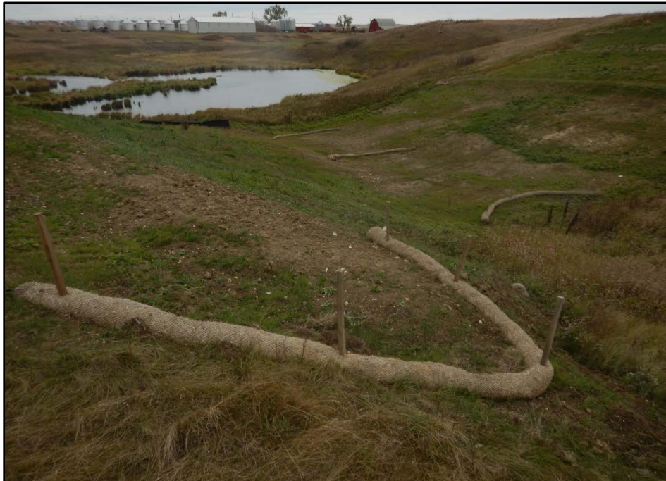
Figure 3. Appearance of ROW along ephemeral drainage. Water bars were established, grass had been planted (August), straw waddles were in place, and silt fencing was maintained at toe slope above the wetland.
