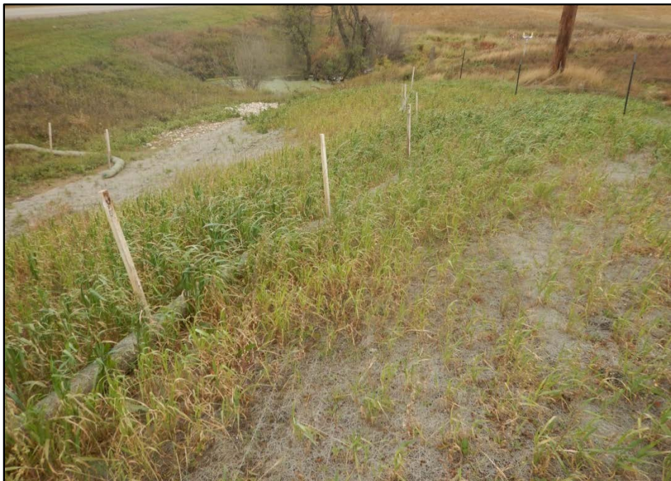
Figure 4. Reclamation in east ditch of Highway 40. Directional drilling equipment was sataged in this area. Seeding, fiber matting, straw waddles, and rock rip-rap have been placed adequately to secure the disturbed slope.
