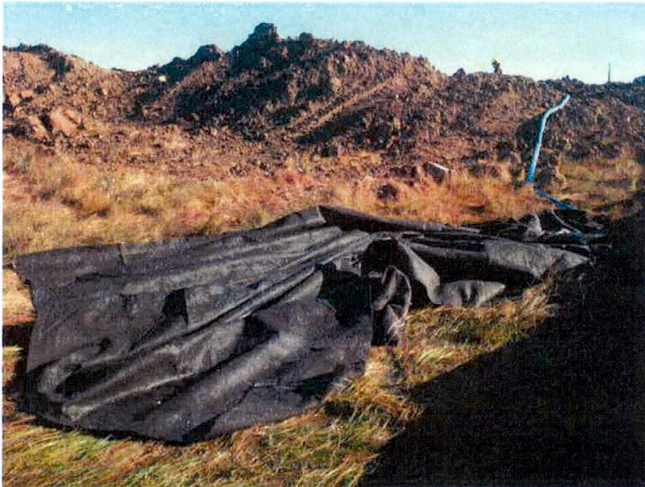
September 20, 2013 - Dewatering into sediment bag contained within a heavily vegetated grassland area
