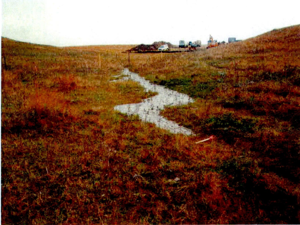
Mud and water release at directional bore site under cultural area at MP 74.98.
