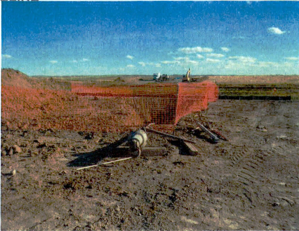
End of directional bore at MP 56.79, prior to pulling pipe back through bore.
