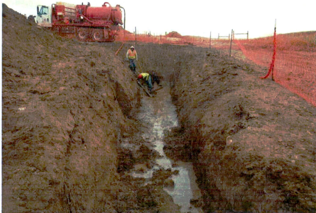
Removal of mud and water at the end of directional bore started at MP 59.19.
