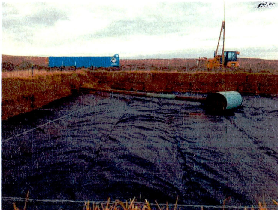
Discharge water containment area with dissipater
