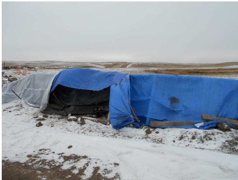
Photo 8 – Block valve #6 at pipeline crossing of ND Highway 85.
