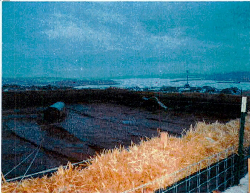
MP 30.91 Discharge energy dissipation structure following discharge. Note abundant iron precipitate.
