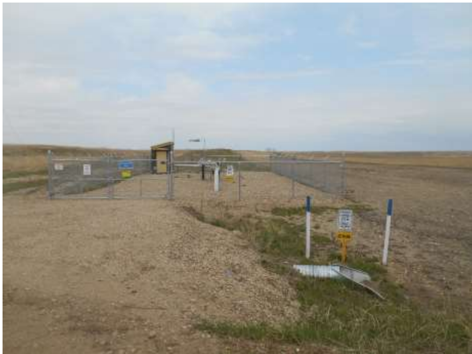
Photo 2 – 011: Typical mainline block valve station
