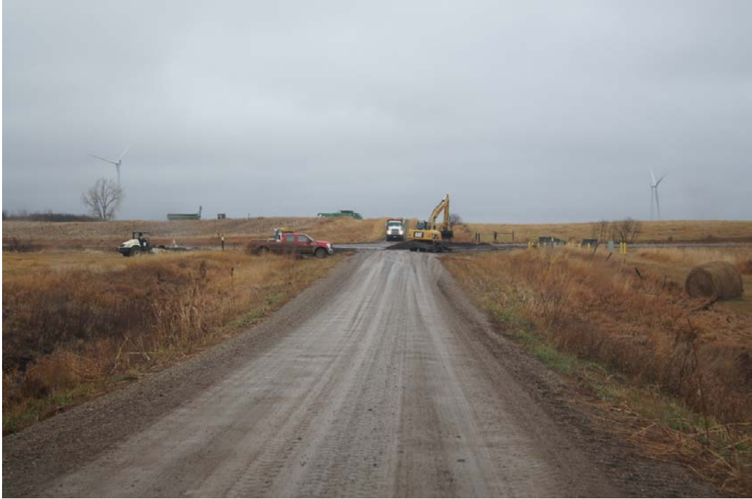
Road radius reduction at road corners, this road was a crane traveled road.
