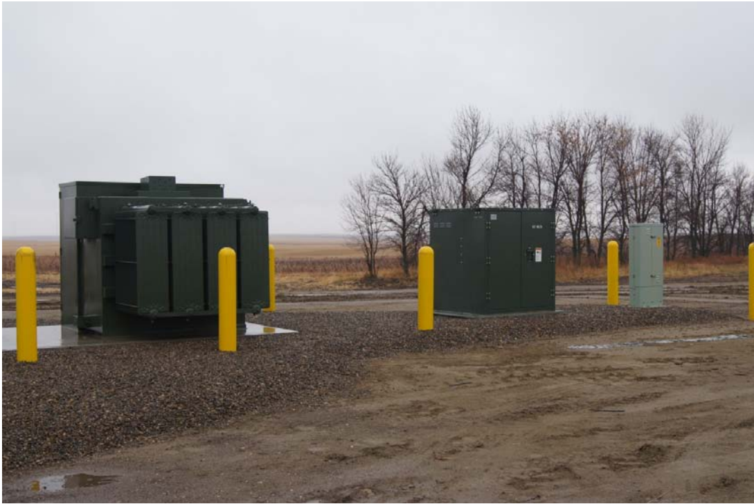
Turbine transformer, collector system switch pedestal, and communication switch pedestal
