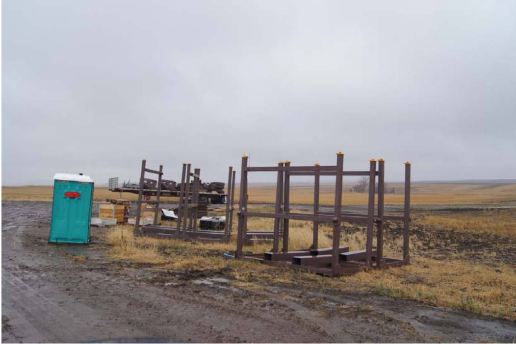
Construction related debris to be removed, portable bathroom.
