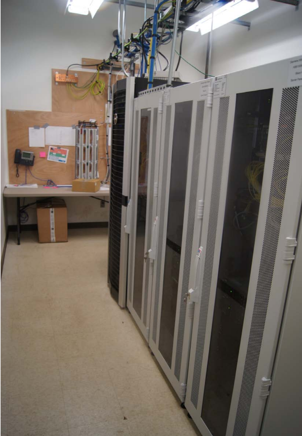
SCADA control room hardware enclosures
