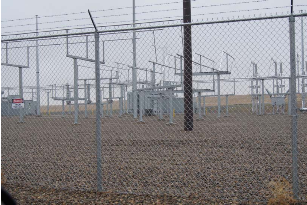
Bison 3 Substation Bay within Bison substation – fencing, Danger high voltage fence signs
