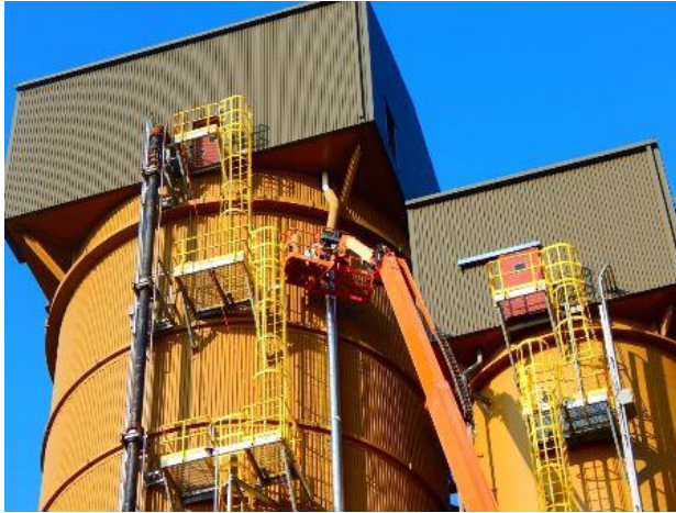
2014-12-09 Siding waste ash silo
