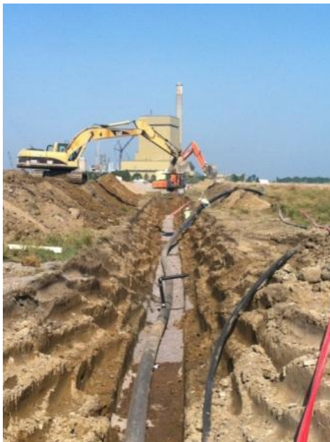
08-15-13 Low quality water line
