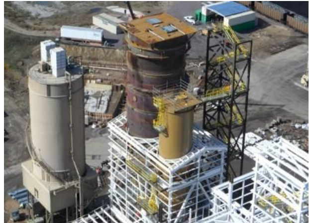
10-07 Waste ash/pebble lime silos
