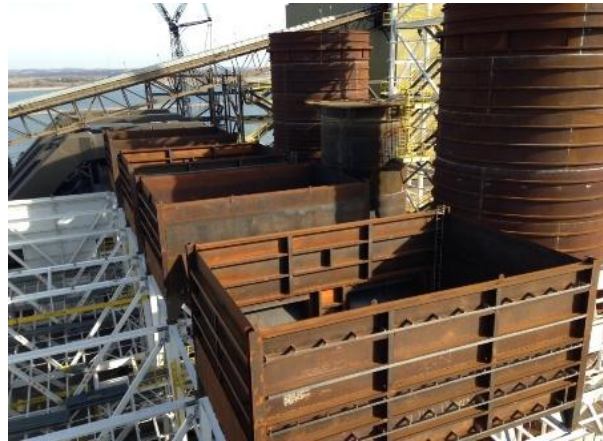
11-04 Lower baghouse modules, hydrated lime silo & scrubber
