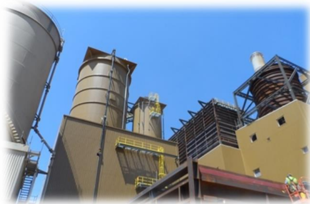
2014-05-22 Waste ash/pebble lime silos
