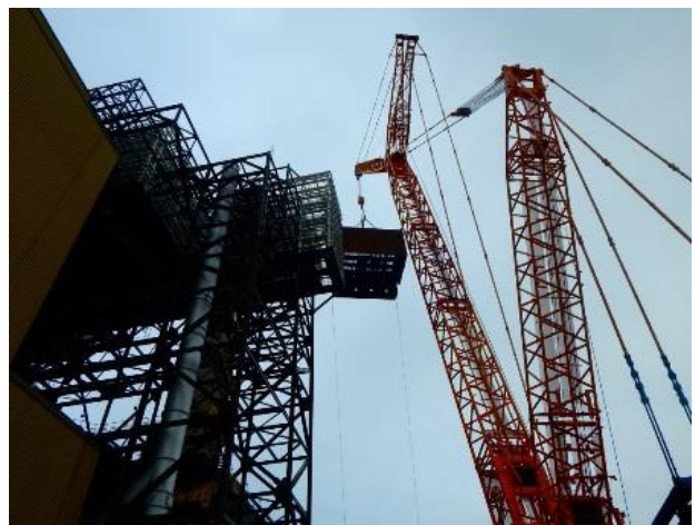
09-04 Reactor box set center SCR
