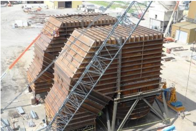
08-04 CFB train 1 and train 2 outlet transition elbows
