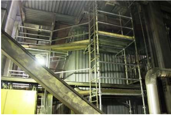
02-11 Staging going on in various areas of the plant in preparation for tie-in outage
