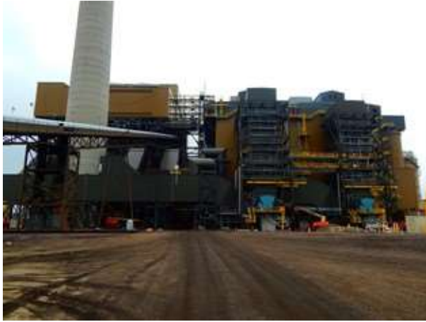
06-02 Baghouse, ID Fans, SCR
