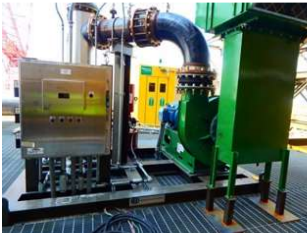
05-27 SCR ammonia layup heater
