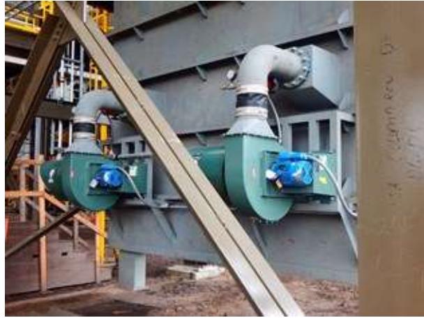
06-02 Damper seal air blowers
