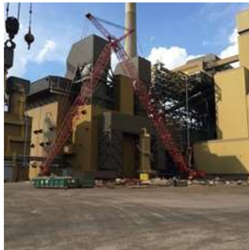
06-07 CFB/baghouse, SCR, corner PL silo
