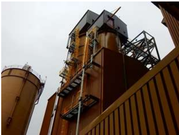
06-02 Waste ash/pebble lime silos
