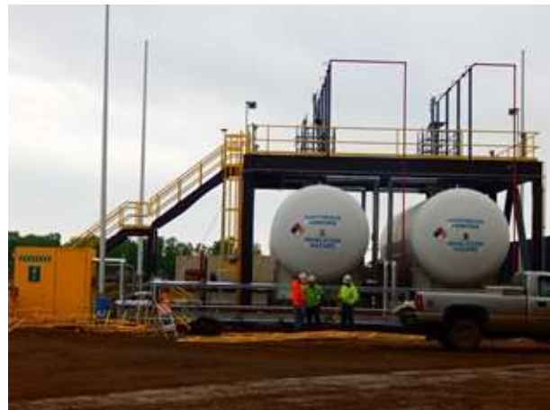
06-03 Ammonia unloading & storage
