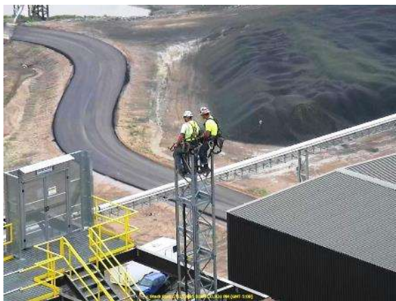
06-11 Taking a break while working to disassemble the construction elevator – 220 feet above ground! They removed a section at a time.
