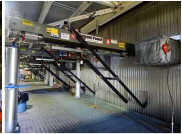
05-27 SCR sootblowers and sonic horns
