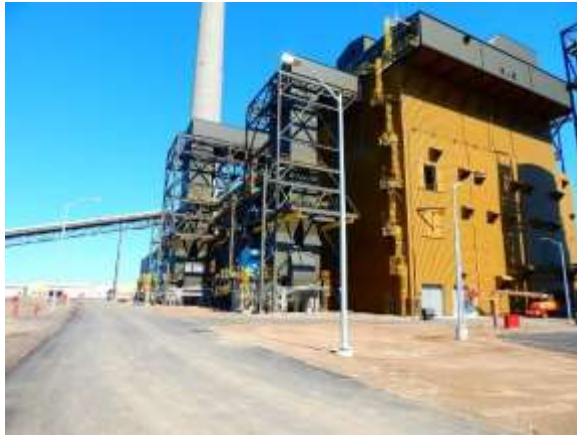
08-20 Baghouse & ID Fans
