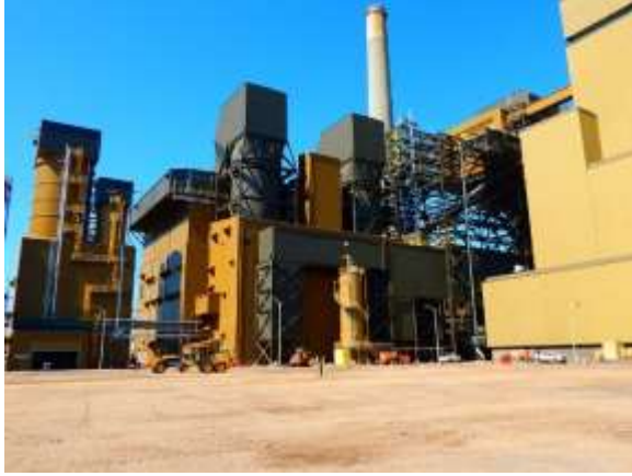
08-20 Waste ash/pebble lime silos, baghouse, CFB, SCR, ACI silo
