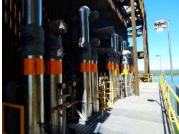
08-20 Ammonia injection grid
