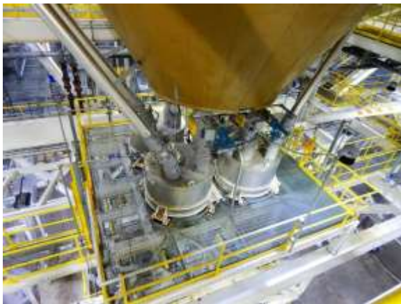
08-20 Hydrated lime weigh bins
