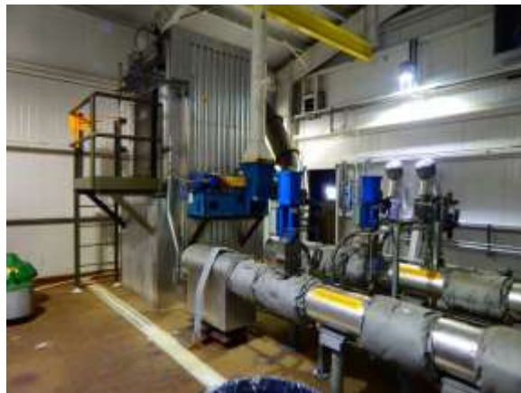
08-20 Hydrated lime system silo dust collector
