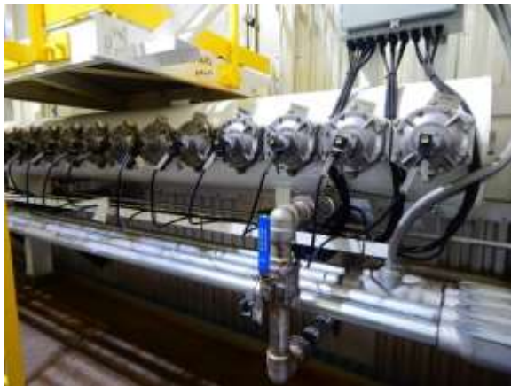
08-20 Baghouse pulse headers
