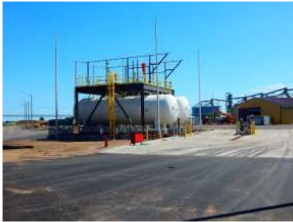
08-20 Ammonia unloading & storage
