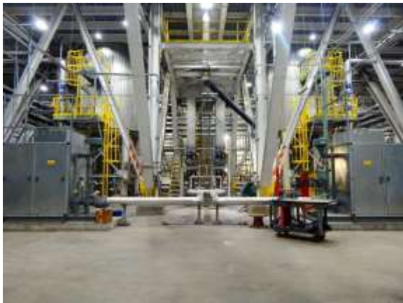
07-07-15 Baghouse process equipment
