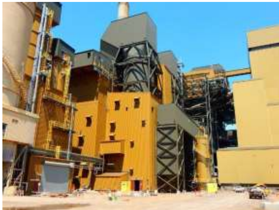
07-07-15 Waste ash/pebble lime silos, CFB, ACI silo and SCR
