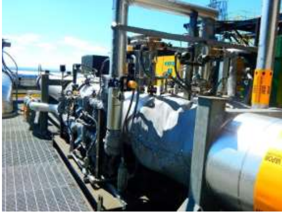
08-20 Ammonia mixing skid
