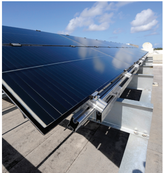
On the roof of its corporate offices in Juno Beach, Fla., NextEra Energy is testing an array of new solar energy technologies for cost-efficiency. Pictured here is thin film technology from MiaSolé.
